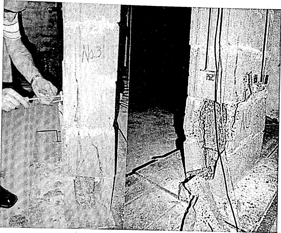
Figure 5.1. Vertical cracks at the block shells of column C1
