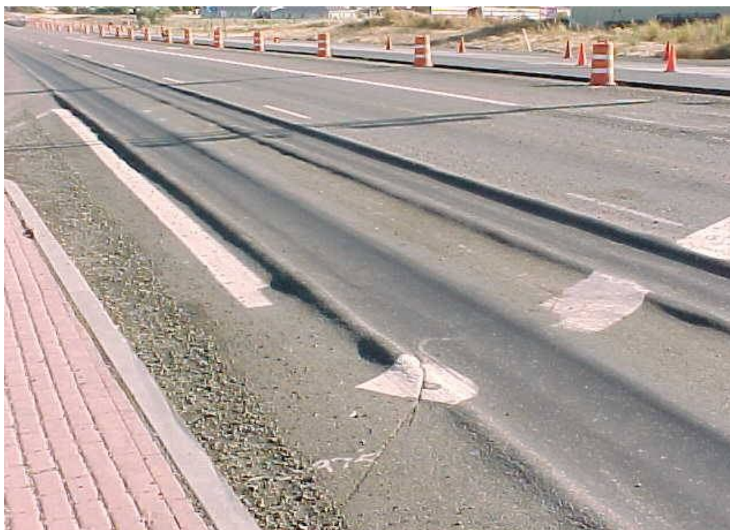
Figure 3.3 High Severity asphalt rutting on highway
