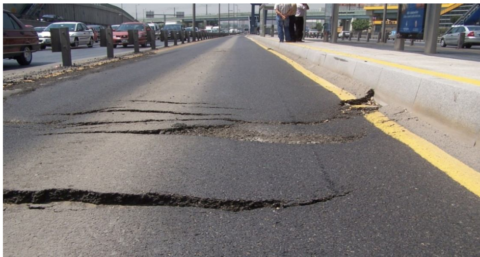
Figure 7.4. Permanent Deformation on METROBUS Line Surface
