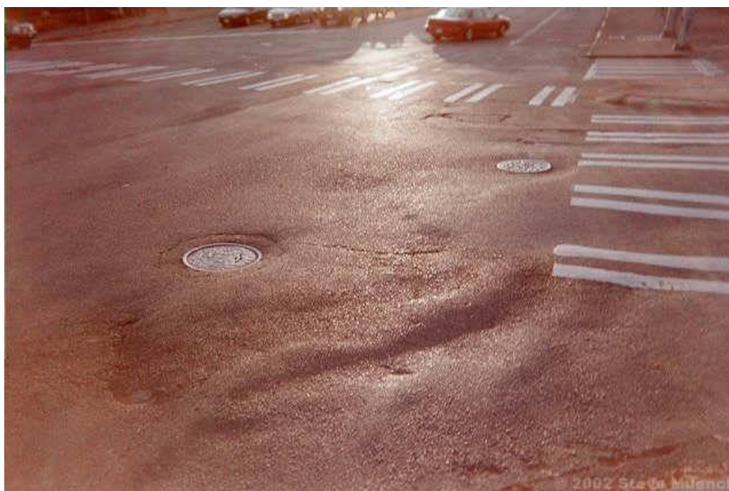
Figure.3.2 Shoving and corrugation on pavement surface
