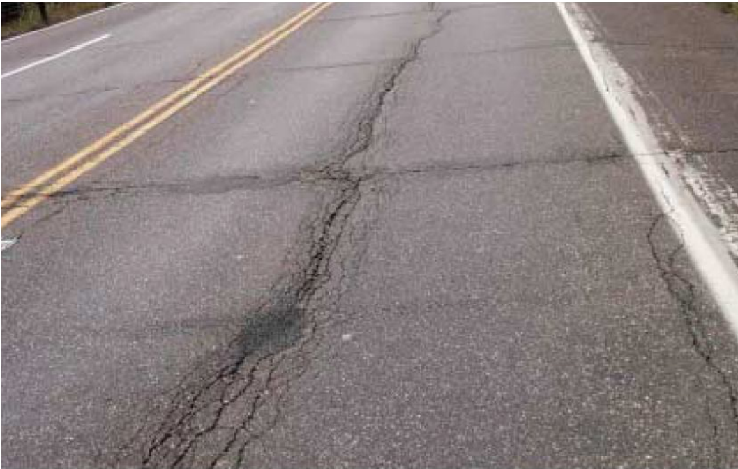
Figure 3.1. High severity longitudinal and transverse cracks.
