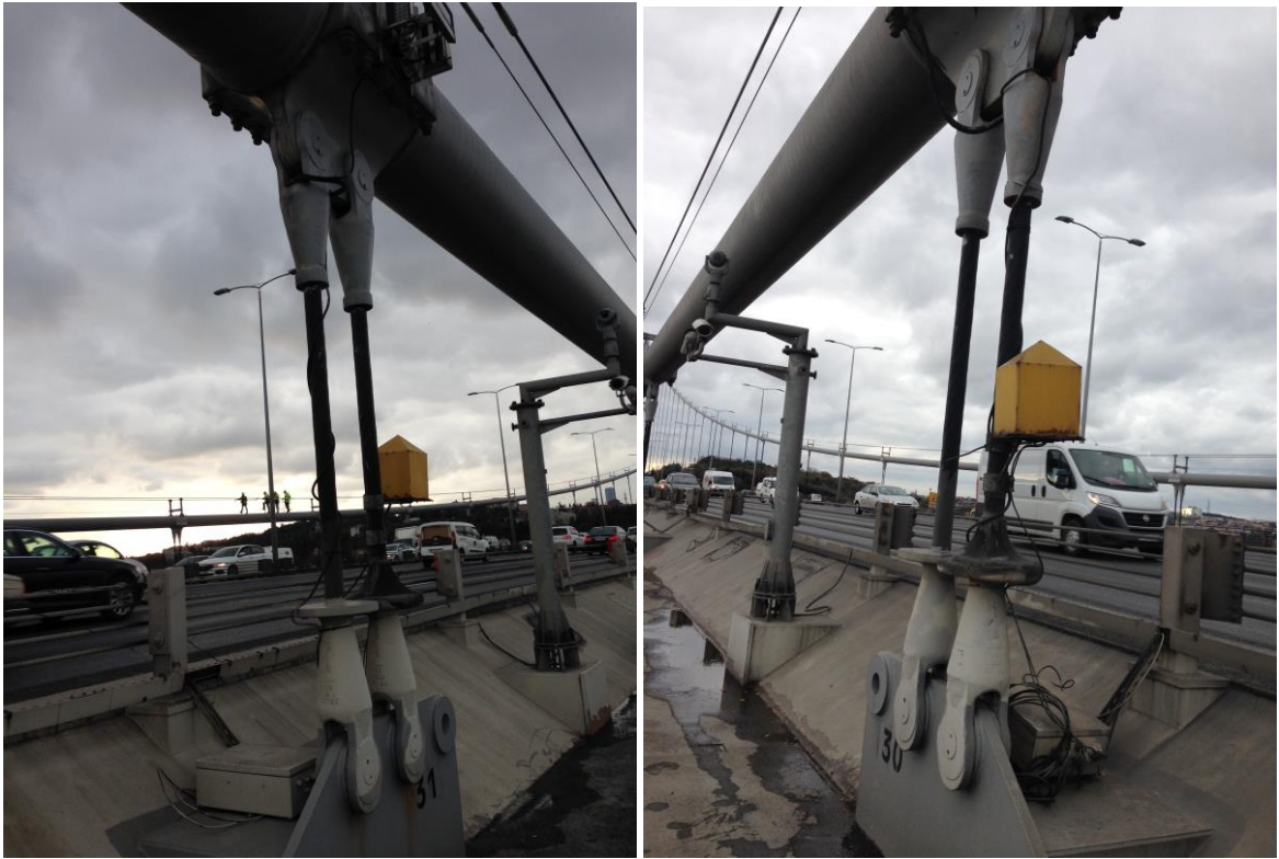
Figure 2.10. Permanent position of sensors on the main span cables (number 11-12).
