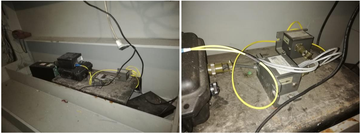
Figure 2.12. Permanent sensor inside the Europe tower, South leg (number 16).
