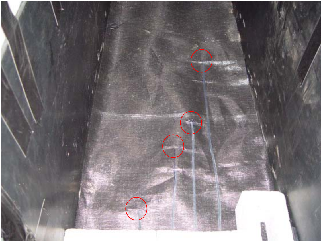
Figure 7.21. The geotextile layer and the regions where the monofilament lines were attached.
