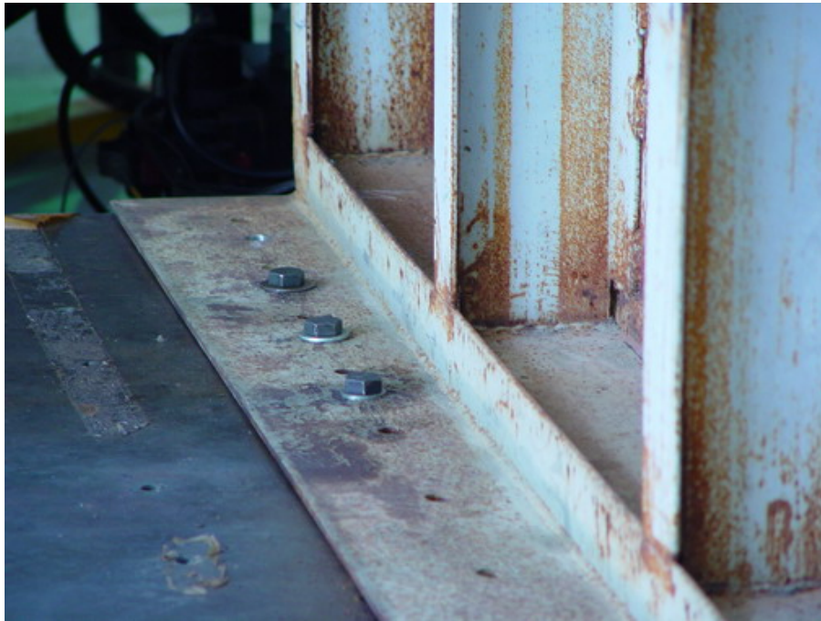
Figure 7.18. 3 of the 8 bolted connections on one side of the steel container. There were 8 connections on the other side as well.
