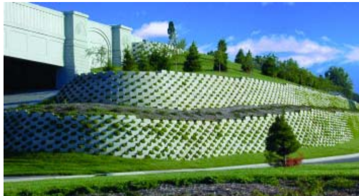
Figure 2.2. A simple illustration of a Geosynthetic-Reinforced Segmental retaining wall (Mirafi Construction Products)
