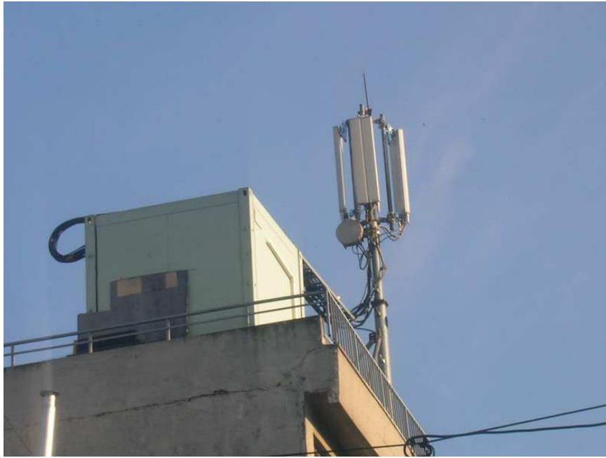
Figure 7.7. Beşiktaş Node B antenna and cabinet
