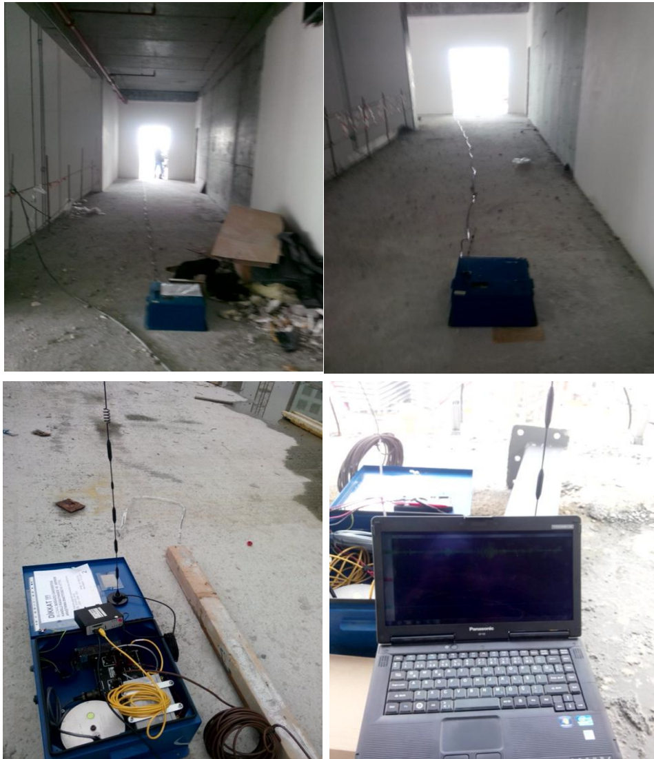
Figure 4.4. Experimental set-up located on the first basement, 7 th and 15 th story (Case 2)
