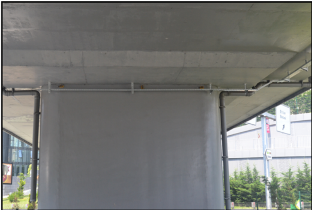
Figure 2.6. Sensors located on the second column.
