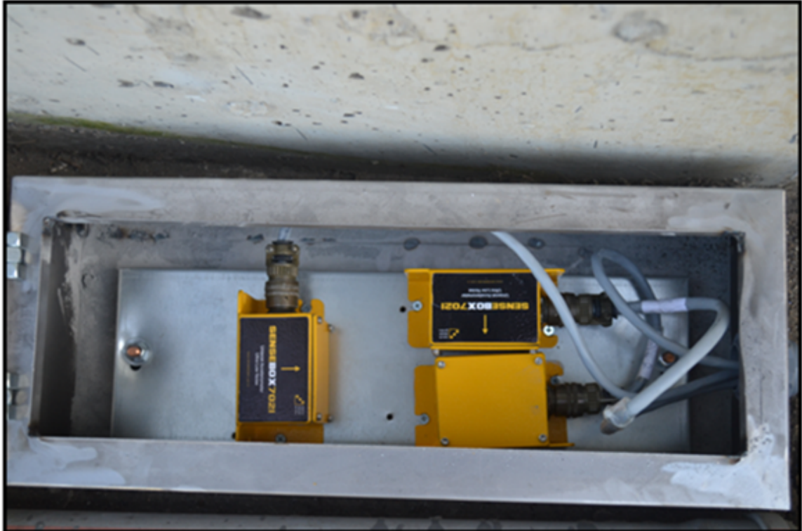
Figure 2.4. Sensors located at the ground level.
