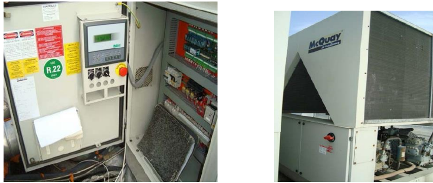
Figure 4.9. (a) Ozone friendly gases in use. (b) Central air conditioning.
