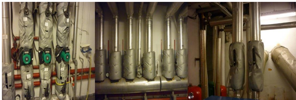
Figure 4.6. Isolation of the valves wrapped with insulating material.
