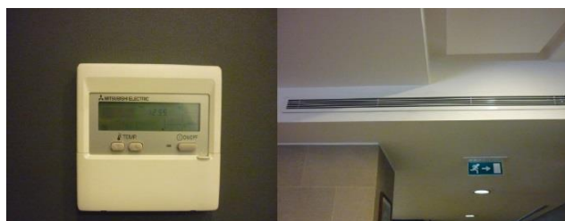
Figure 4.11. Mechanical ventilation system on the floors.
