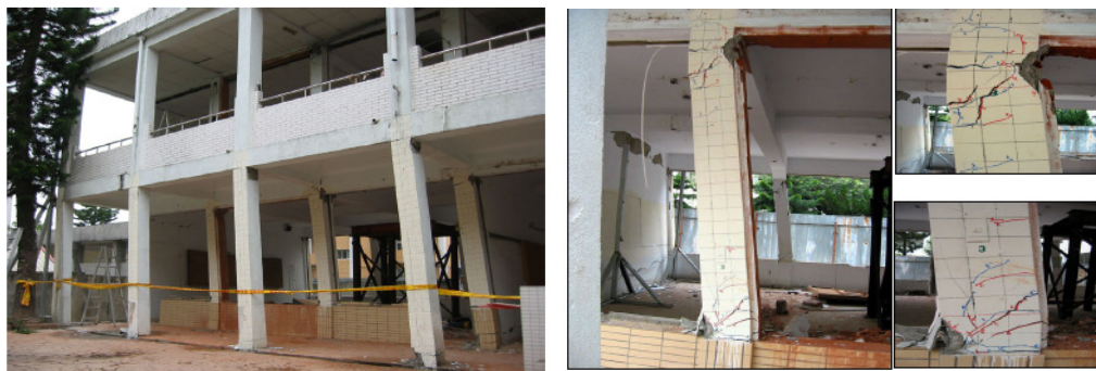
Figure 4.3. Flexure failure (left hand side) and flexure-shear failure (right hand side) of the test building [1]
