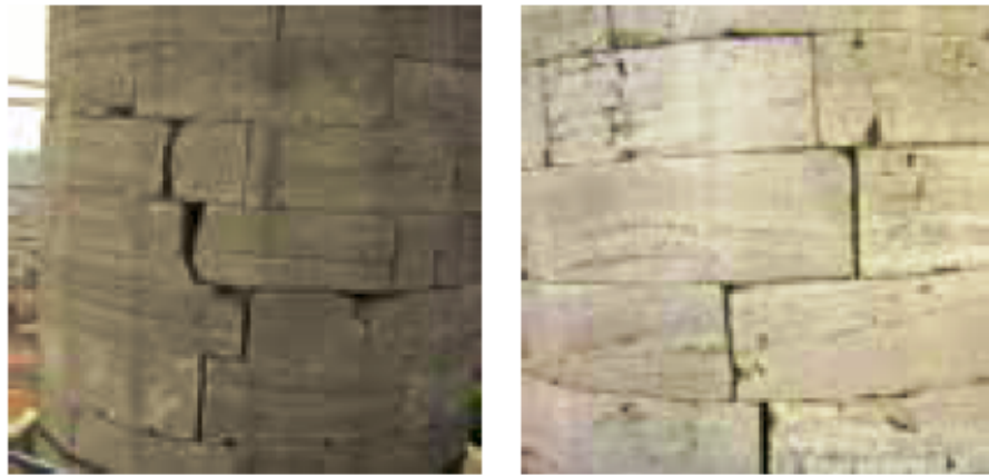
Figure 2.4. Separations in the minaret's stone
