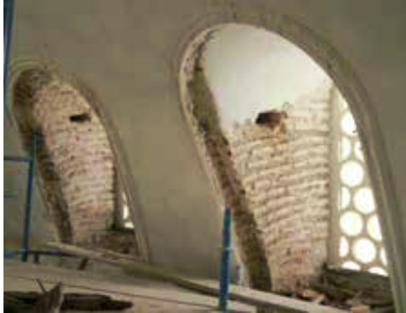
Figure 2.7. The disfunctional timber tie beams
