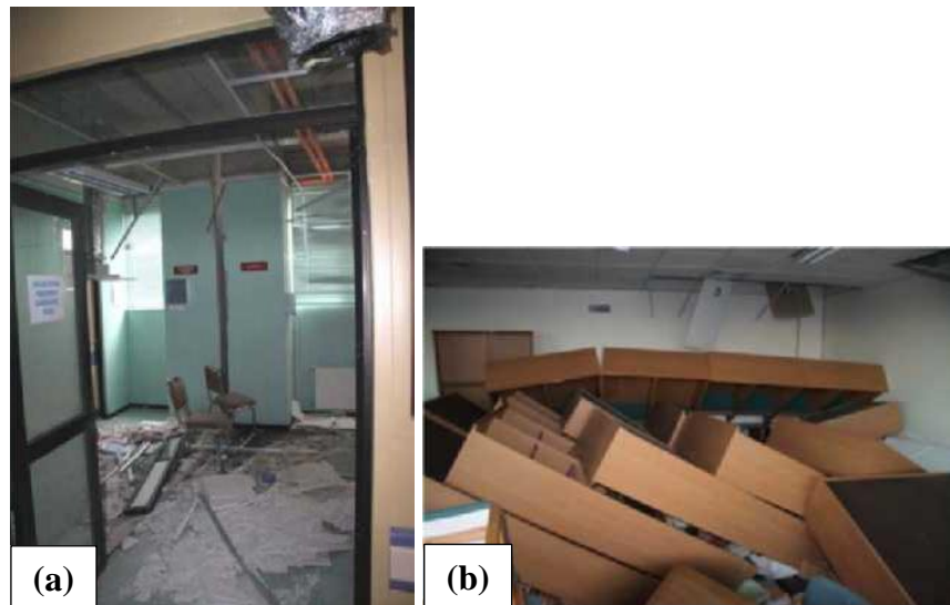
Figure 1.1. Nonstructural damage: (a) fallen ceiling tiles at the San Carlos Hospital and (b) content damage in Talca court house (Miranda et al., 2012) permission in APPENDIX B.
