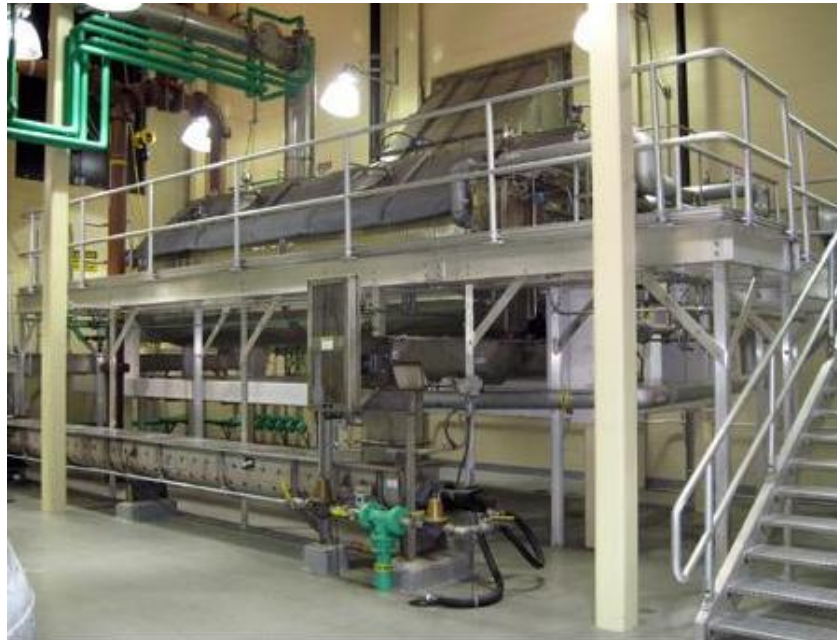
Figure 3.17. Sludge Drying Unit of Paşaköy WWTP
