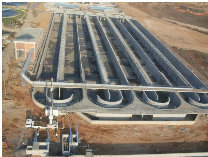
Figure 3.9. Aeration Tanks of Paşaköy WWTP
