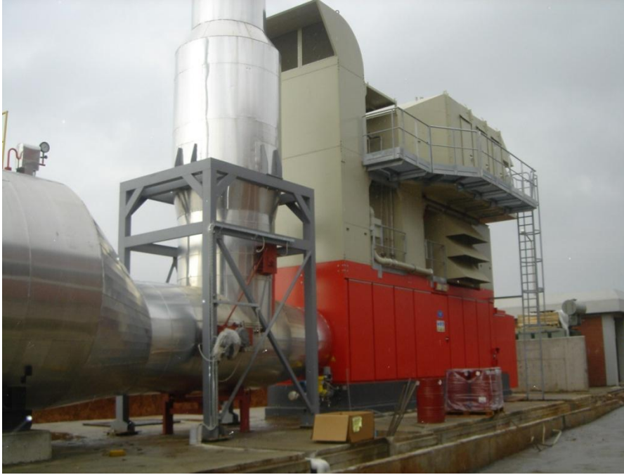
Figure 3.18. Co-Generation Unit of Paşaköy WWTP
