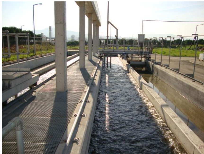
Figure 3.5. Aerated Grit Chambers of Paşaköy WWTP
