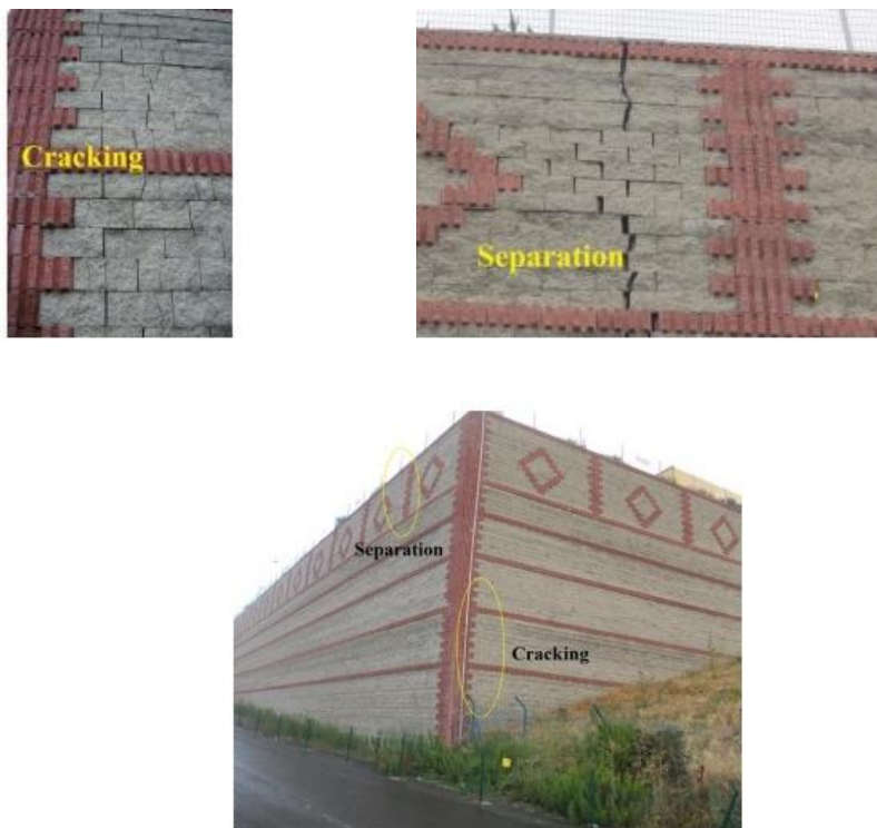
Figure 1.5. Discrepancies observed in a typical GRS wall structure with corner turns from Hamderi and Guler (2015).
