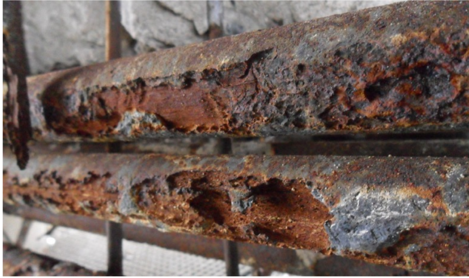
Figure 2.3. Effects of corrosion on reinforcement.
