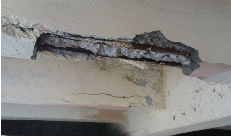
Figure 2.7. Concrete spalling due to corrosion.
