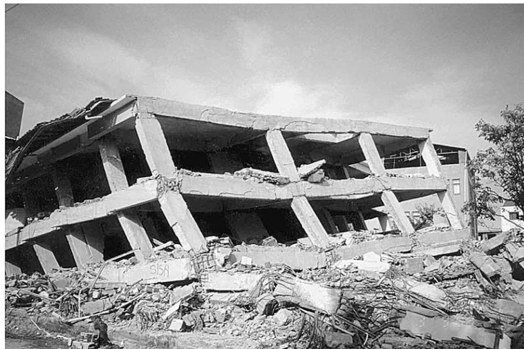
Figure 2.6. Joint Failure (El-Amoury and Ghobarah 2002)
