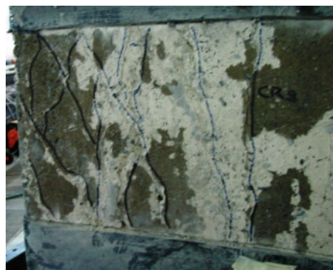
Figure 4.11. Image of the joint after the removal of FRP wraps
