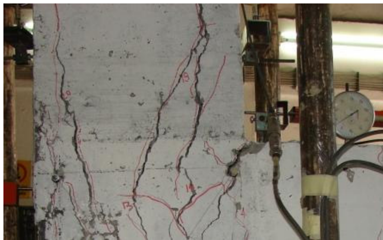
(a) Top column shear cracks
