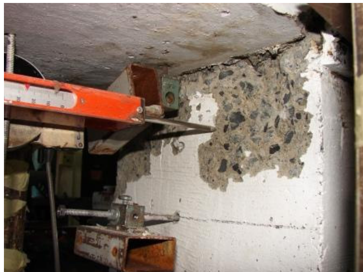
(b) Bottom column damage due to slippage
