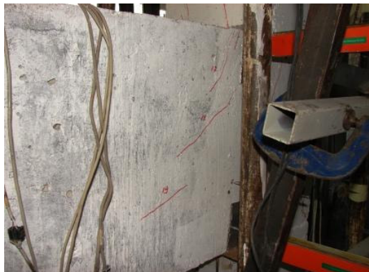
(c) Diagonal cracks at the backside of the transverse beam (2.75% drift level)
