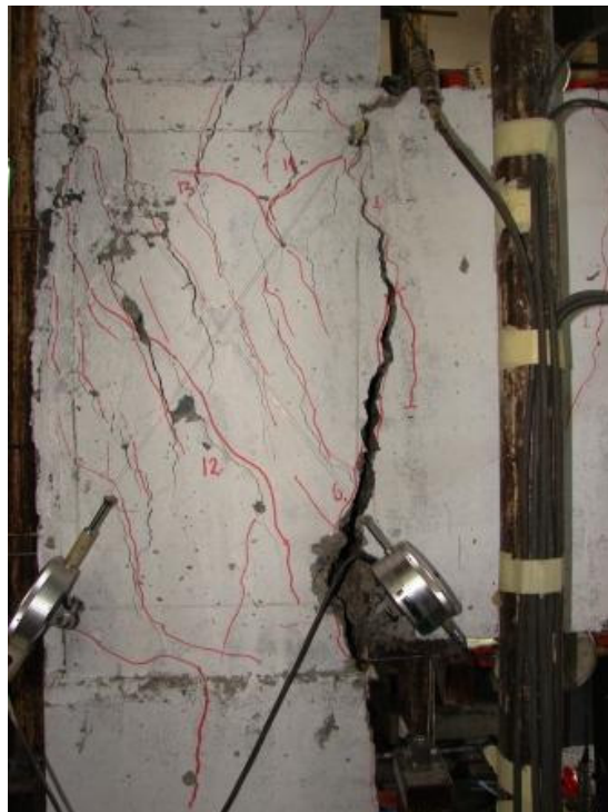
(b) Crack Pattern of US3-C-Control in push direction of loading
