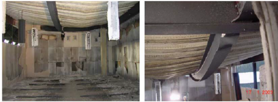
Figure 2.4. Displaced Geometry of Composite Floor System Tested in Cardington Fire Test-7 (Vassart and Zhao, 2011).
