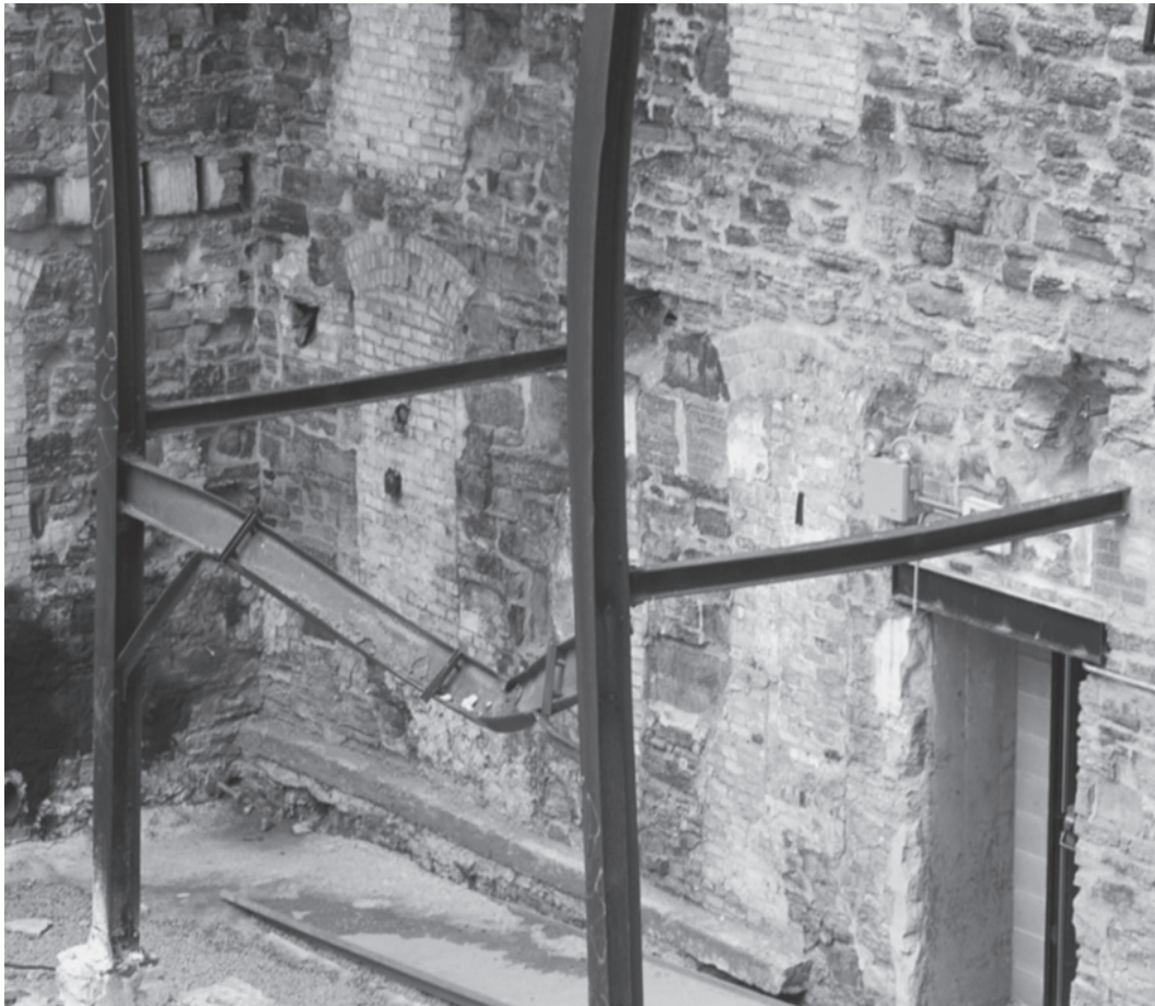
Figure 1.3. Lateral Torsional Beam Buckling Exaggerated by Fire.
