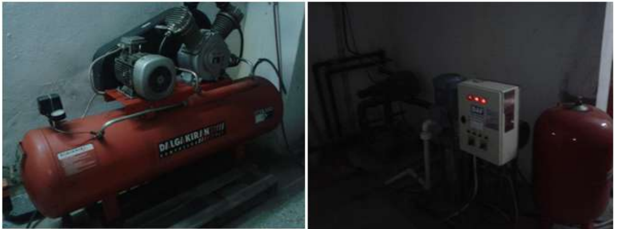
Figure B.27. Compressors and boilers.
