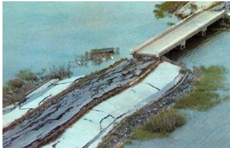
Figure 5.11. Slumping of a road embankment (Towhata, 2008).
