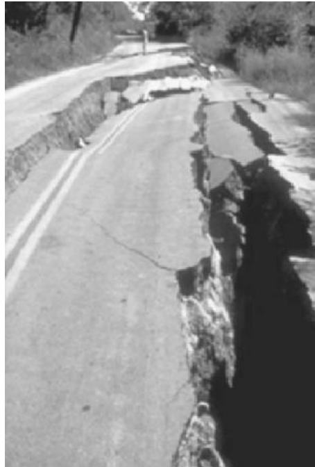
Figure 2.8. Earthquake induced damage after the 1989 Loma Prieta Earthquake (Day, 2002).
