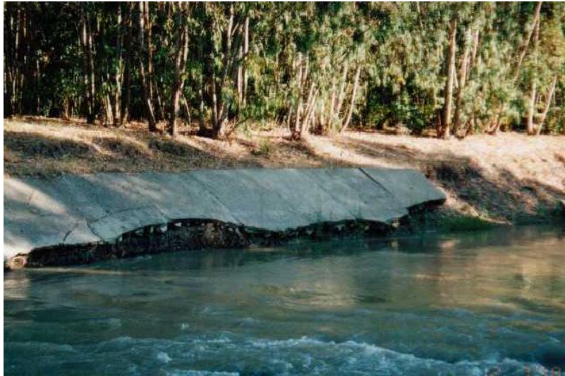
Figure 5.8. Collapsed river bank located on the failed embankment (Japan Society of Civil Engineering Reports, 1998).
