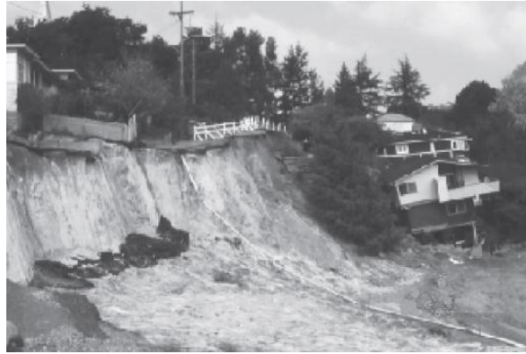
Figure 2.2. The London Road Landslide, Oakland, CA (Duncan, 2005).
