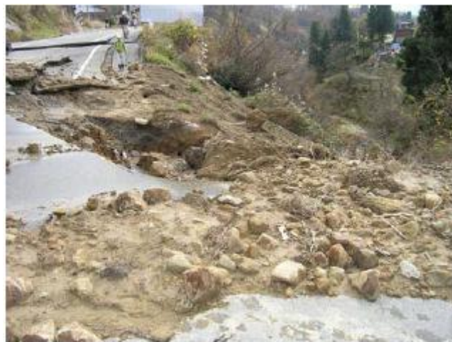
Figure 5.3. A failed road embankment due to sliding failure (Towhata, 2008).
