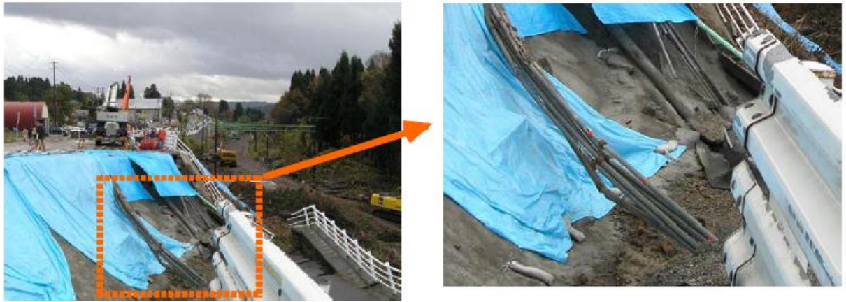
Figure 5.2. A sliding failure of a road embankment and destroyed pipelines after 2004 Niigata-Chuetsu Earthquake (Towhata, 2008).
