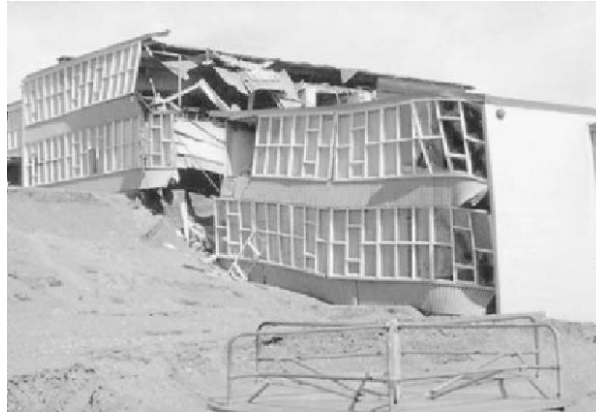
Figure 2.6. Government Hill School damage after earthquake induced slope failure (Day, 2002).
