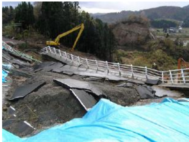
Figure 5.13. Densification damage of a road embankment due to subsidence (Towhata, 2008).
