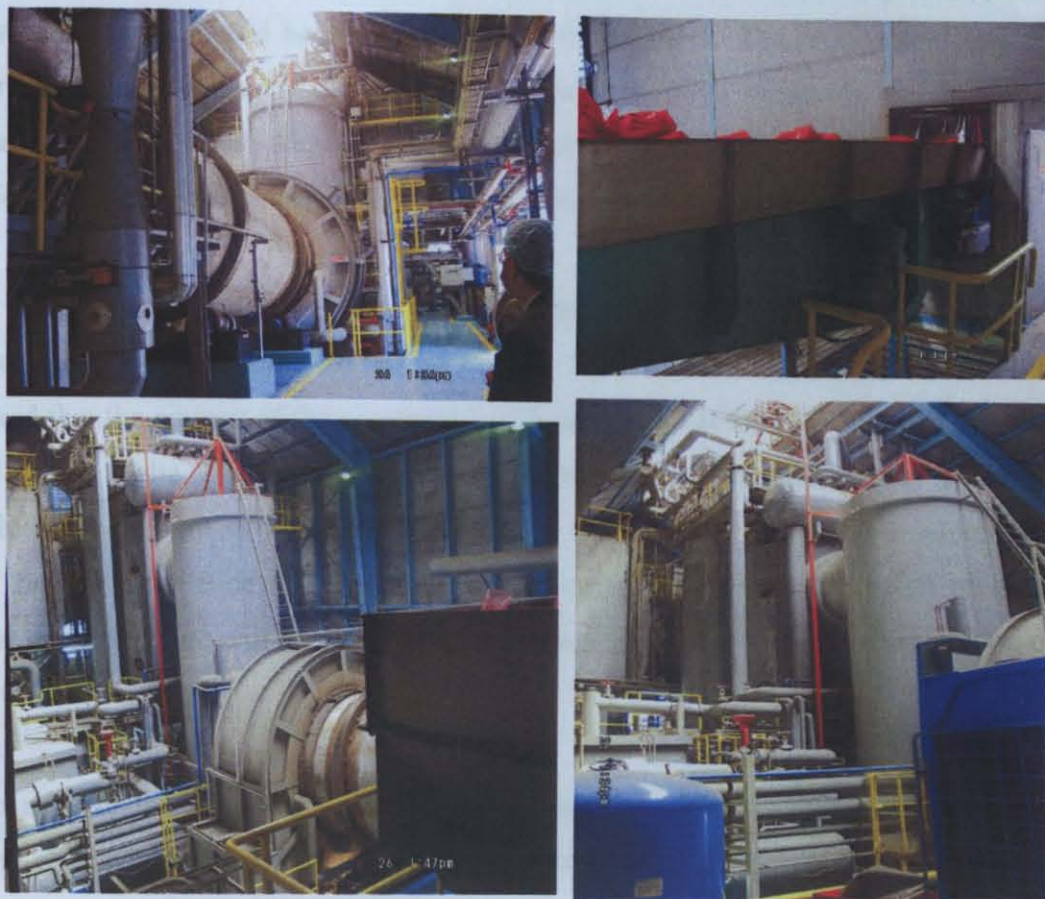
Figure 3.16. The Kemberburgaz-Odayeri Incineration Plant.
