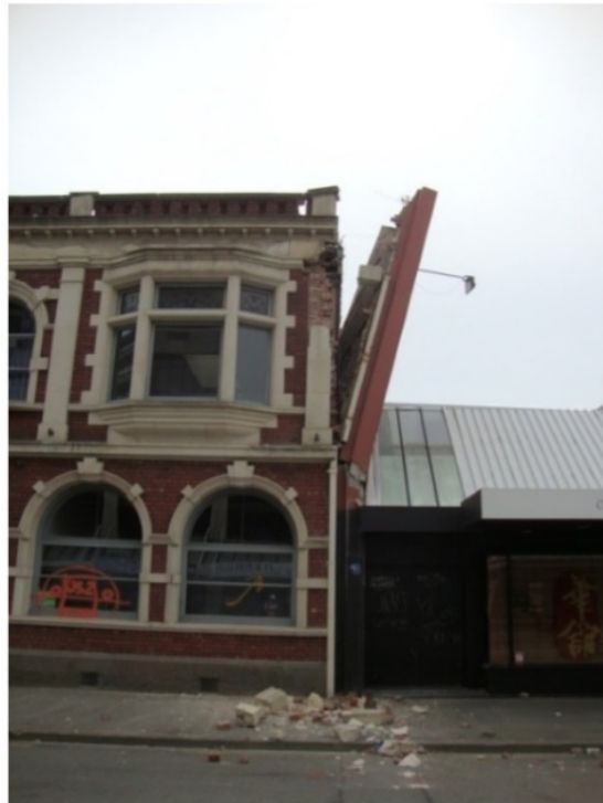
Figure 2.3. Out-of-plane instability of the wall subjected to face load due to a lack of ties between the face-loaded wall and rest of the structure [17].
