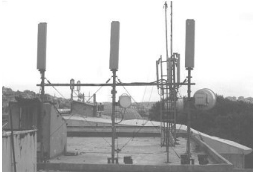
Figure 2.5 Three sector antennas on top of a roof.
