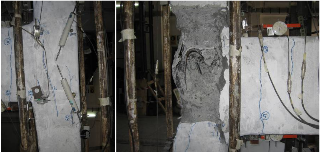
Figure 3.35. Damages of Specimen TR-5-R
