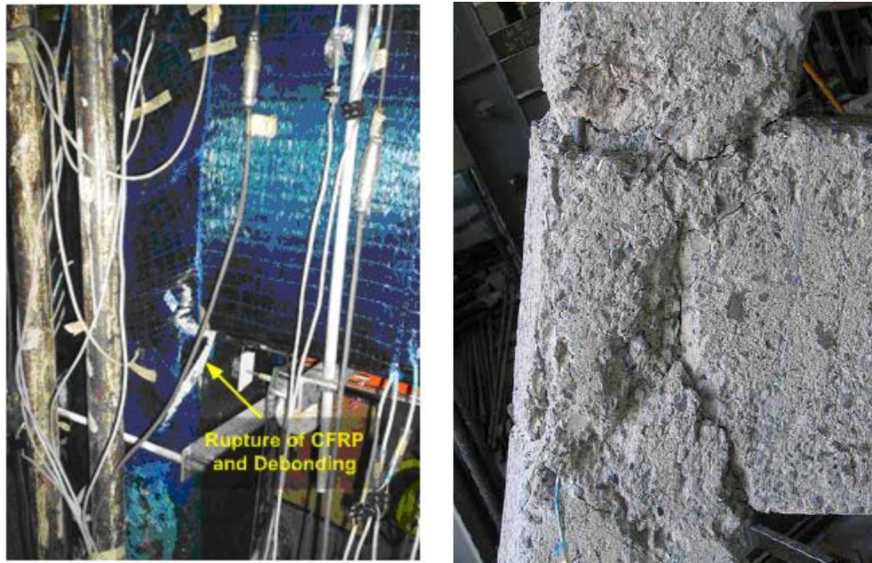
Figure 3.28. Rupture of CFRP and crack pattern of Specimen TR-5-FRP-1
