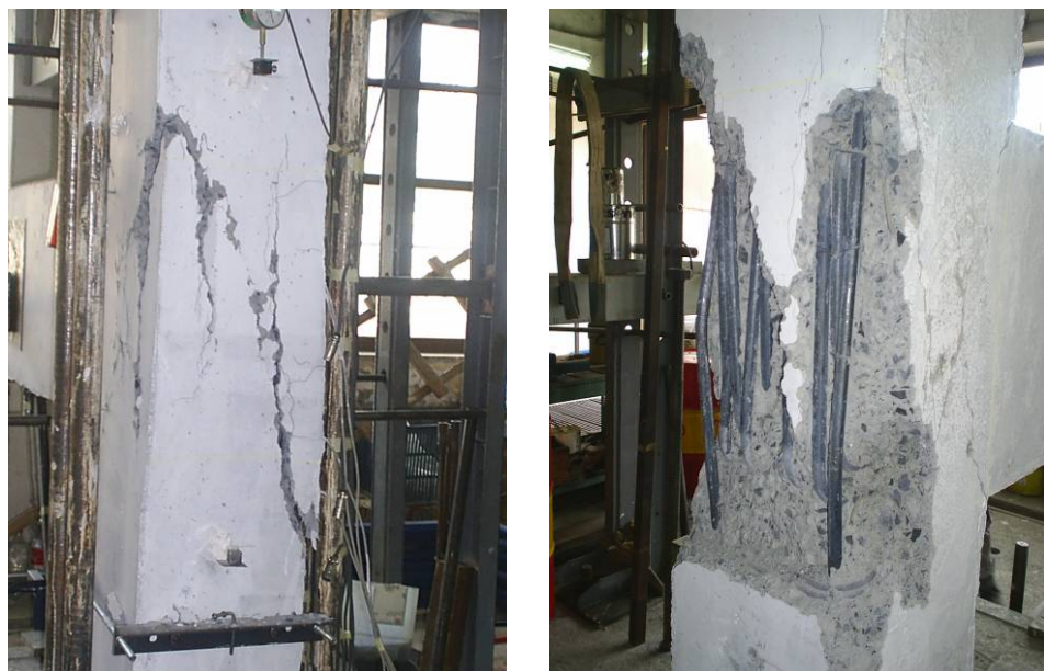
Figure 3.20. Buckling of column reinforcements
