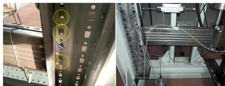
Figure 3.33. Failure Modes of BC140 - Tearing at Tabs.
