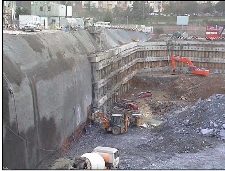
Figure 3.19. Combination of soil nailing with tied-back bored pile application for the deep excavation of BJK Fulya Complex (Zetas, 2006)
