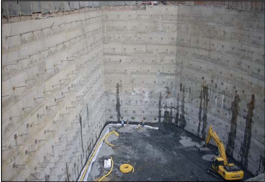
Figure 3.9. Segmented reinforced concrete wall with pre-stressed anchor application for the deep excavation of a hotel building in Istanbul (Zetas, 2006)
