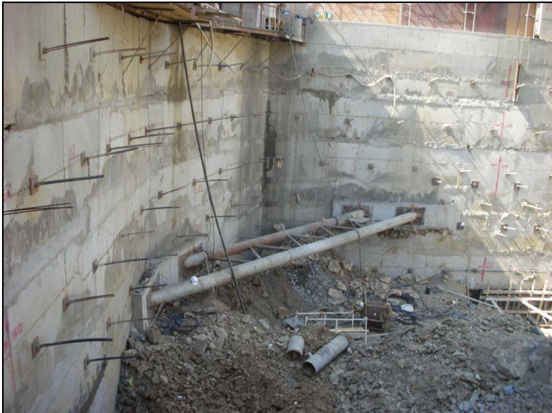
Figure 3.11. Struts used together with pre-stressed anchors for the excavation of a hotel building (Zetas, 2006)
