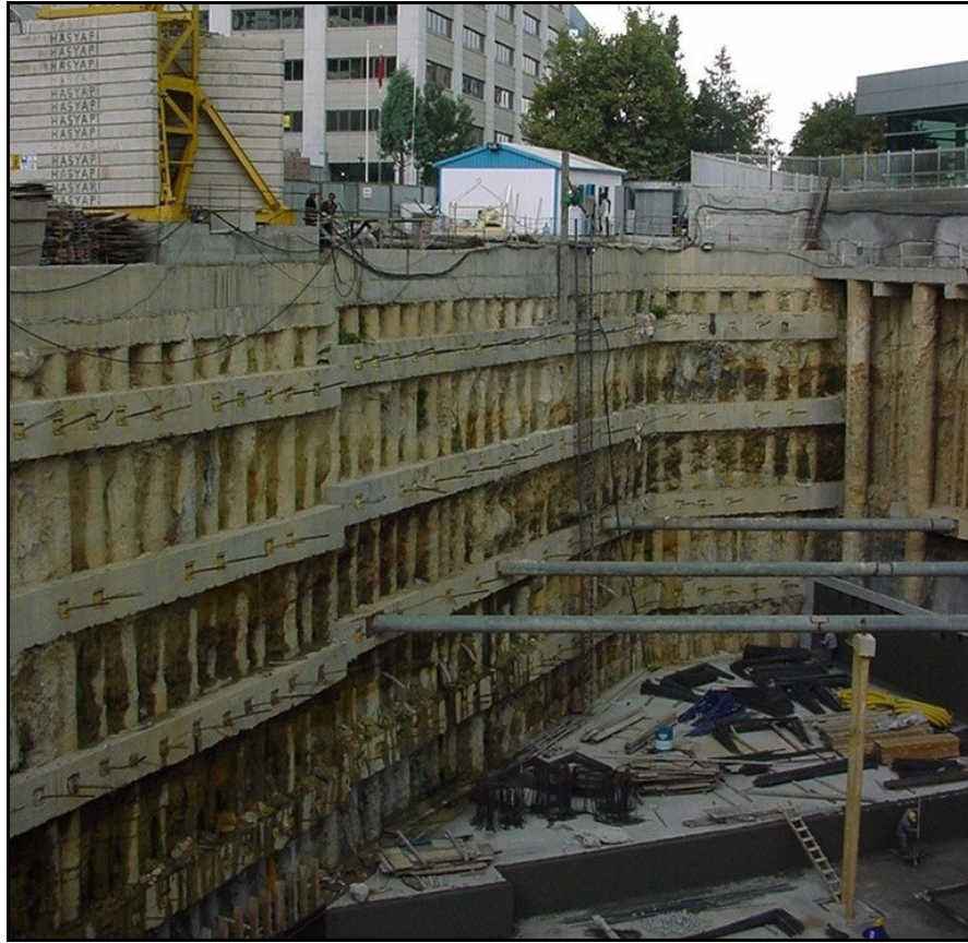
Figure 3.12. Struts used instead of pre-stressed anchors for the one face of a deep excavation in Istanbul (Zetas, 2006)
