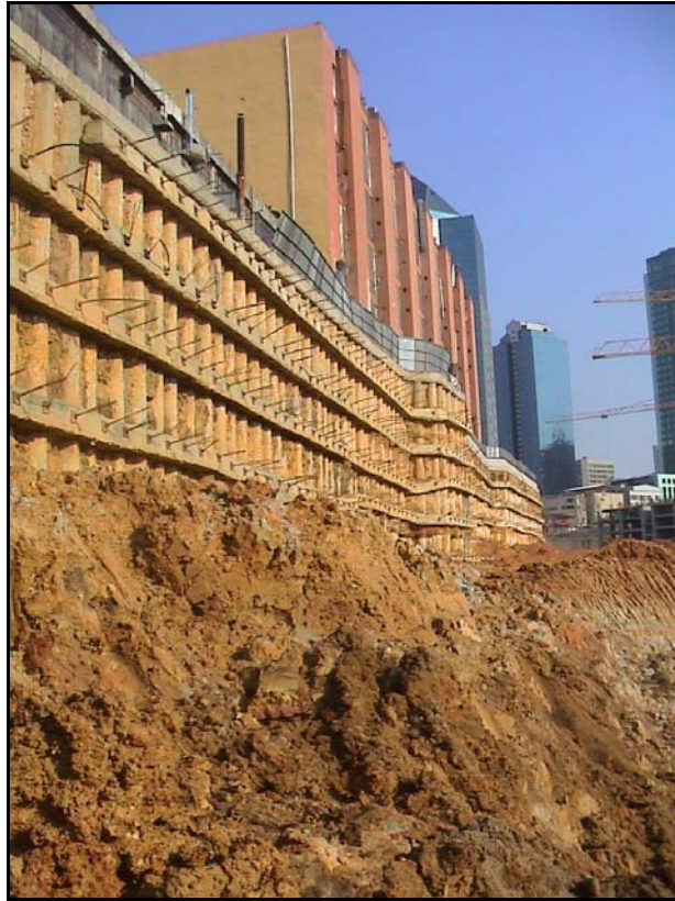
Figure 3.3. Tied back cast in-situ bored pile application on the deep excavation of Mashattan Residence (Zetas, 2006)
