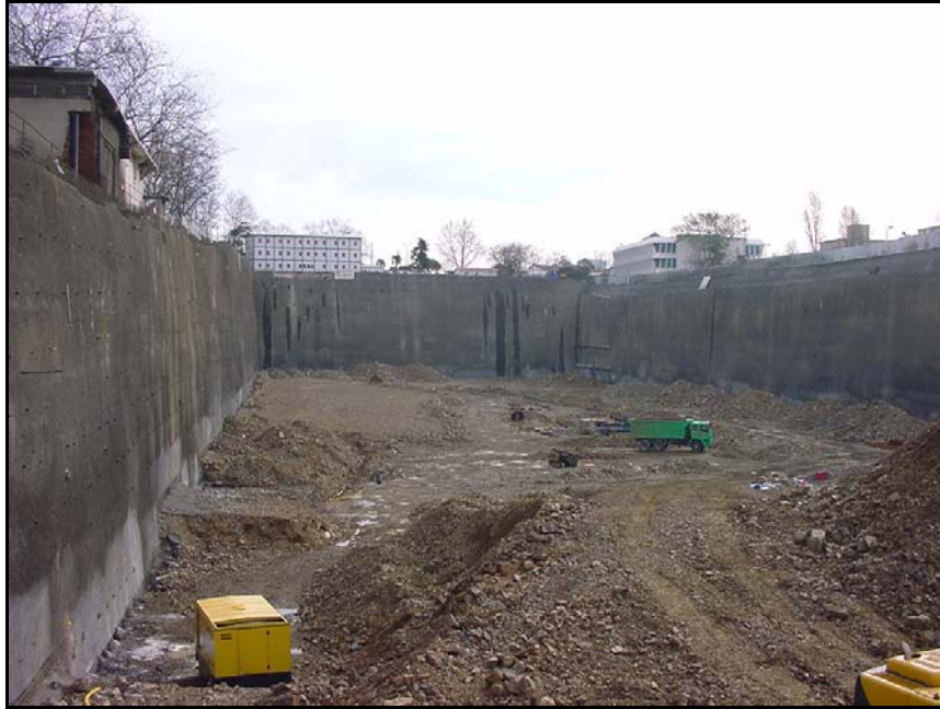
Figure 3.13. Soil nailing used for all faces of the deep excavation of Kanyon Complex (Zetas, 2006)
