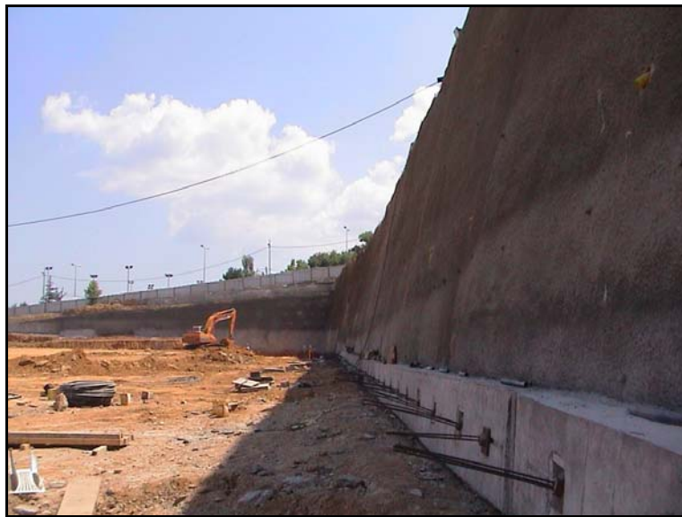
Figure 3.20. Combination of soil nailing with tied-back bored pile application for the deep excavation of Istinye Park Project (Zetas, 2006)
