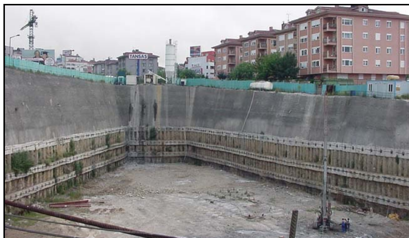
Figure 3.18. Combination of soil nailing with tied-back bored pile application for a deep excavation in Istanbul (Zetas, 2006)
