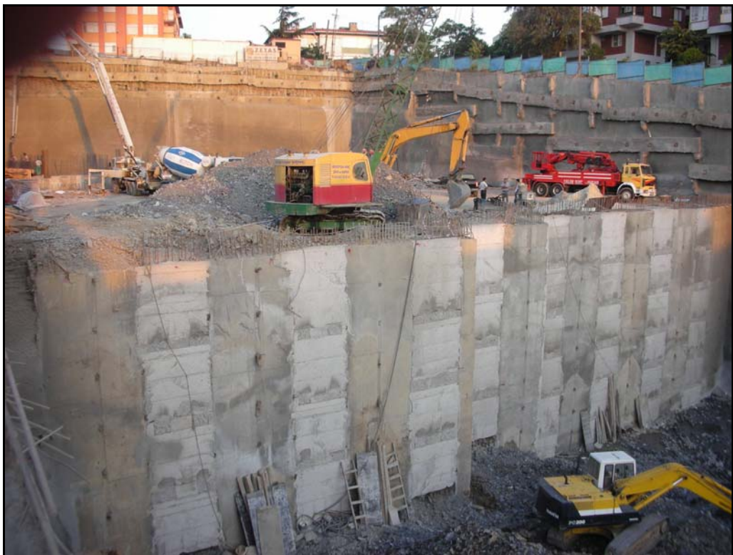
Figure 3.10. Cast in-situ manually dug caisson wall with pre-stressed anchor application for the excavation of a hospital building (Zetas, 2006)
