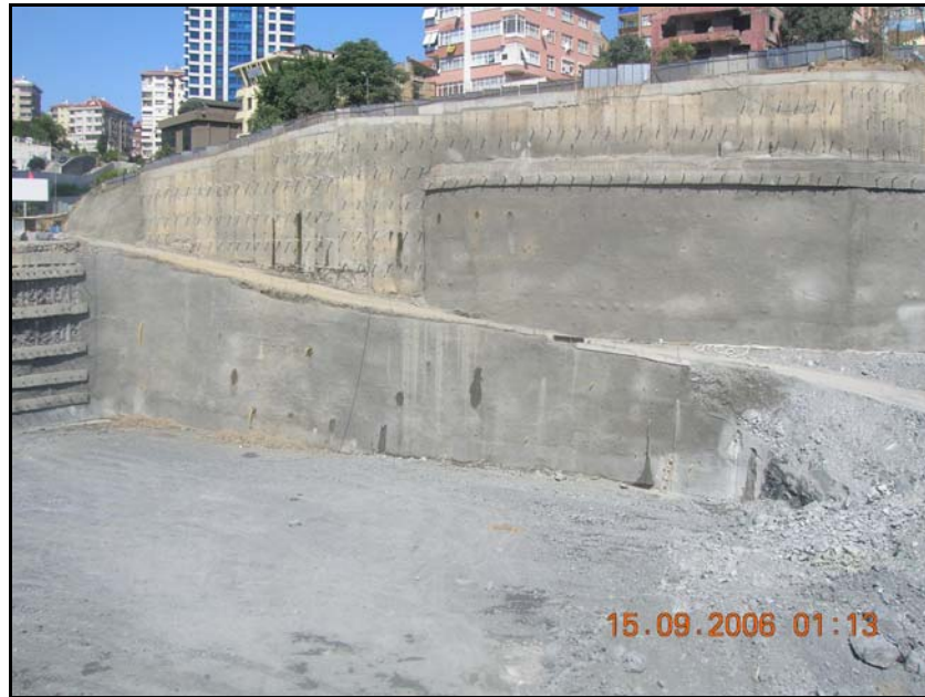
Figure 3.15. Additional one row of pre-stressed anchor at the top to prevent displacement soil nailing in BJK Fulya Complex (Zetas, 2006)
