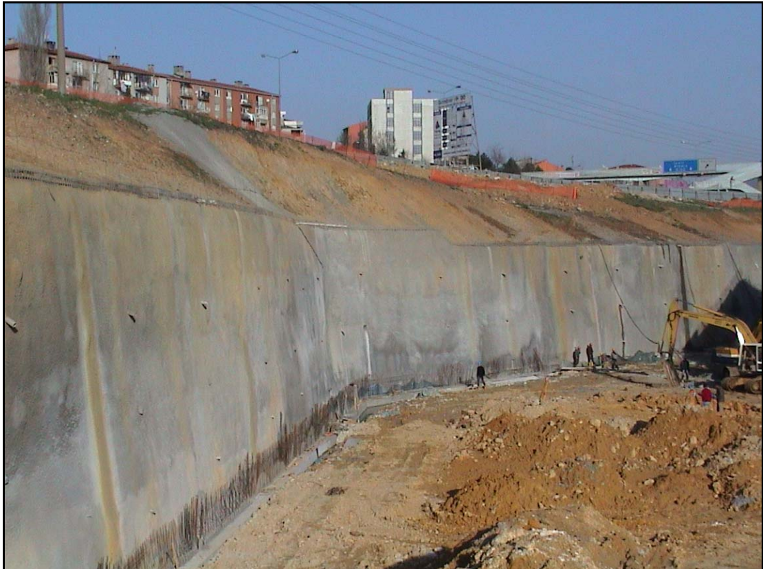
Figure 5.26. A photograph from Tepe Shopping Mall, inclinometer 4 section
