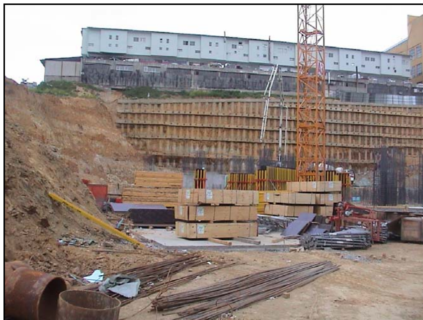
Figure 3.4. Tied back cast in-situ bored pile application on another section from the deep excavation of Mashattan Residence (Zetas, 2006)
