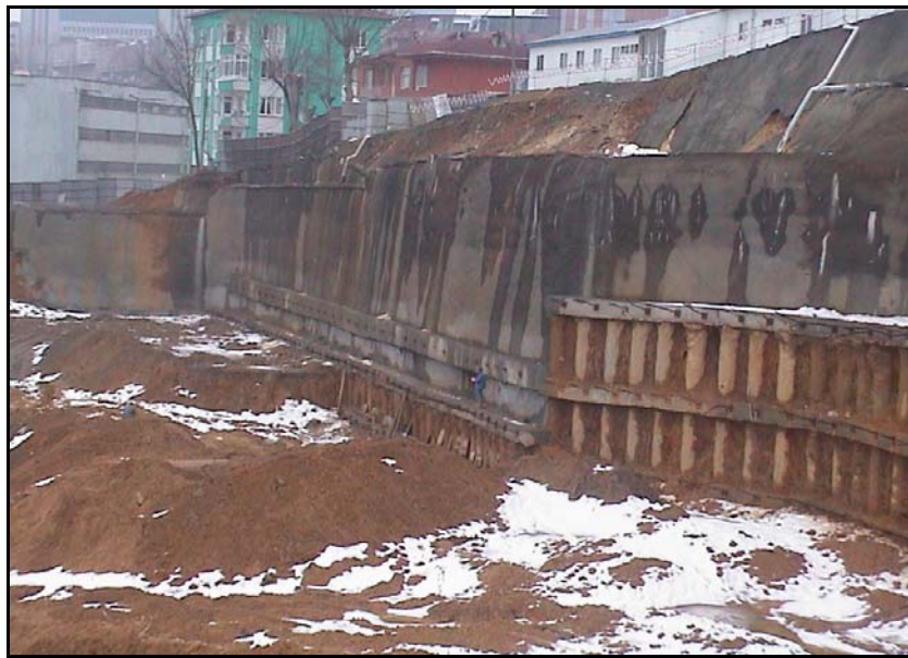
Figure 3.17. Combination of soil nailing with tied-back bored pile application for the deep excavation of Mashattan Residence (Zetas, 2006)
