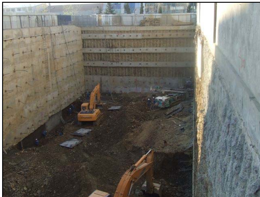
Figure 3.7. Micro piles with pre-stressed anchors applied for the excavation of a building in Istanbul (Zetas, 2006)
