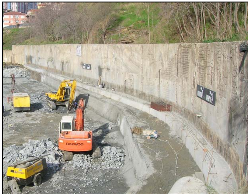
Figure 7.18. Completion of the first row of soil nailing under the existing retaining wall
