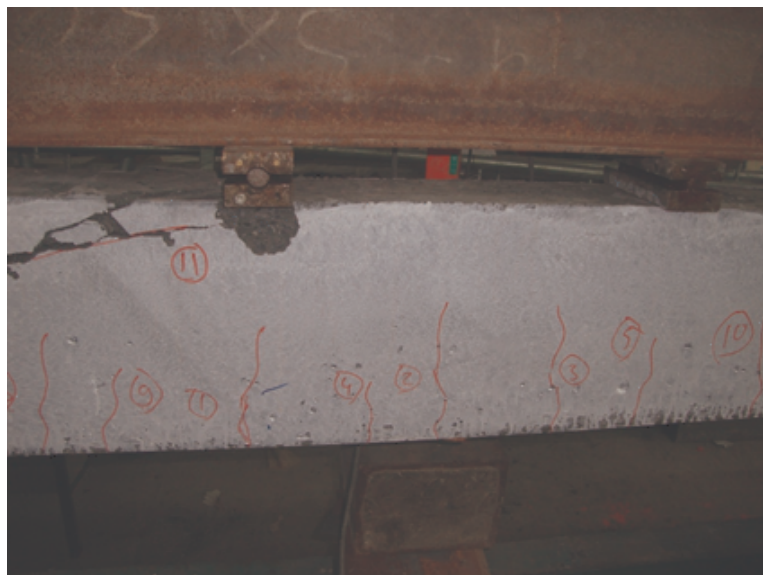
Figure 4.11. Crack propagation of B-04.
