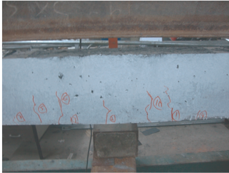
Figure 4.25. Crack propagation of B-09.
