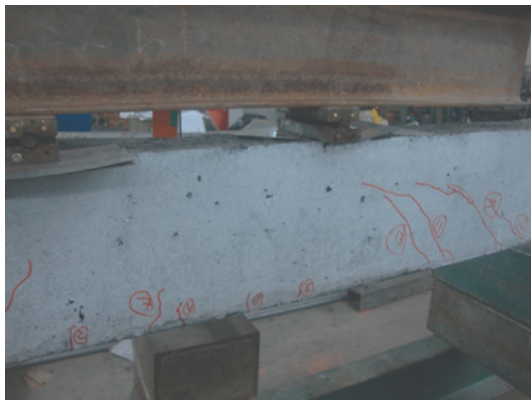
Figure 4.28. Crack propagation of B-10.
