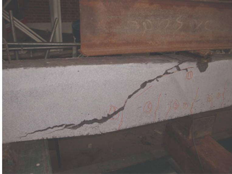
Figure 4.12. Damaged shape of B-043.
