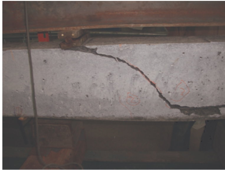
Figure 4.6. Damaged shape of B-02.
