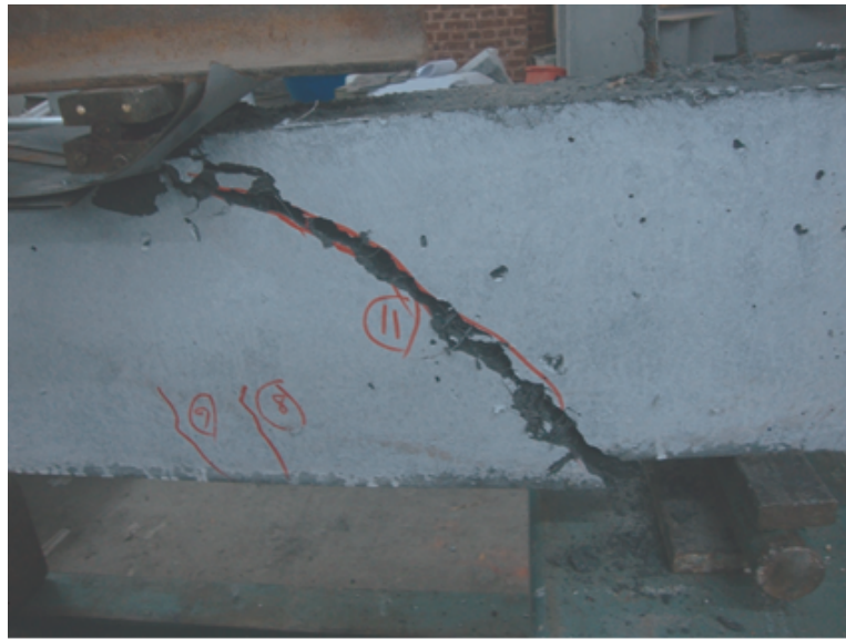
Figure 4.26. Damaged shape of B-09.
