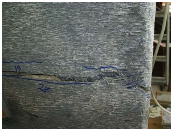
Figure 4.69. Close-up of cross diagonal under the ruptured wrapping overlay
