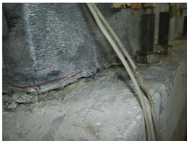
Figure 4.70. Close up of the separation around right column
