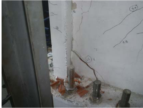
Figure 4.47. Formation of compression strut and formation of crushing around left column
