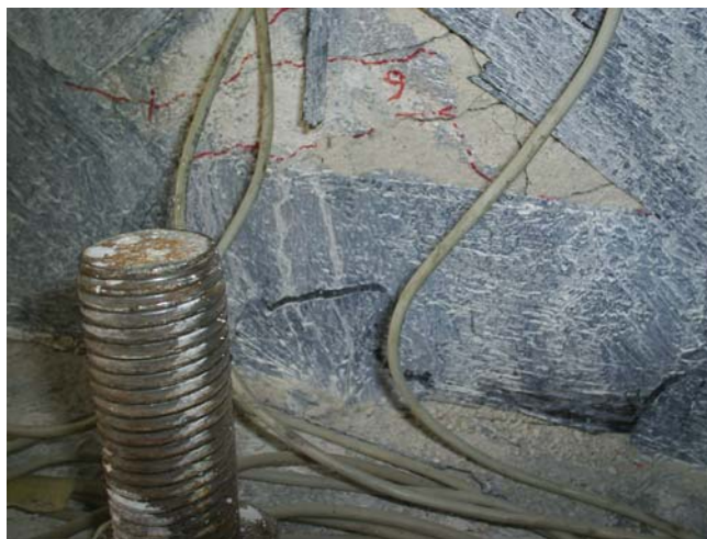
Figure 4.73. Close-up of the anchorage sliding
