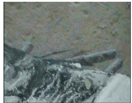
Figure 4.34. Close-up of anchorages around left column at the end of the test
