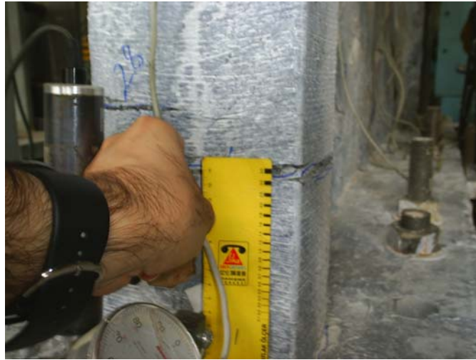
Figure 4.68. Close-up of a crack width on the left column outer face
