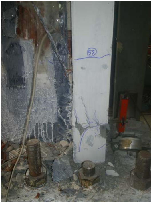
Figure 4.41. Close-up of the right column bottom end
