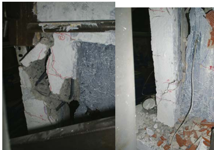
Figure 4.62. Close-up of left column top and bottom ends
