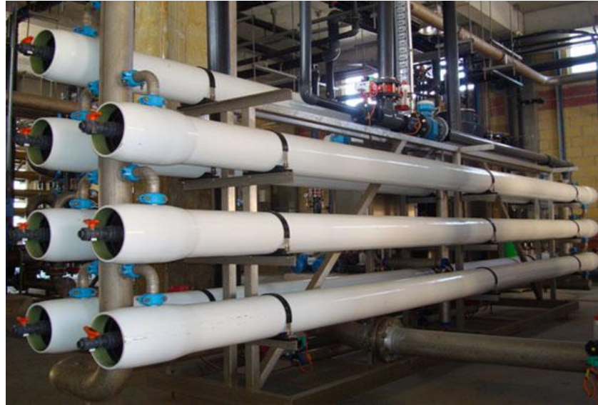
Figure 7.12. Nano filtration capillary membranes (İSTAÇ, 2010)
