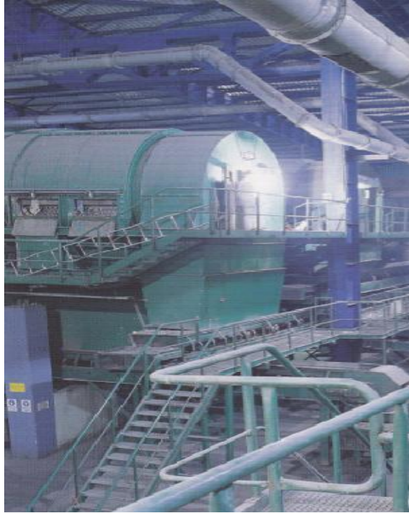
Figure 7.14. Kemberburgaz Compost Facility (İSTAÇ, 2010)
