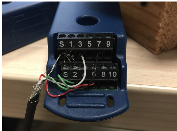
Figure 3.12. Load cell cables attached to a NI-9949 module.
