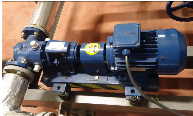
Figure 4.11. Installed internal gear pump on ORC test rig.
