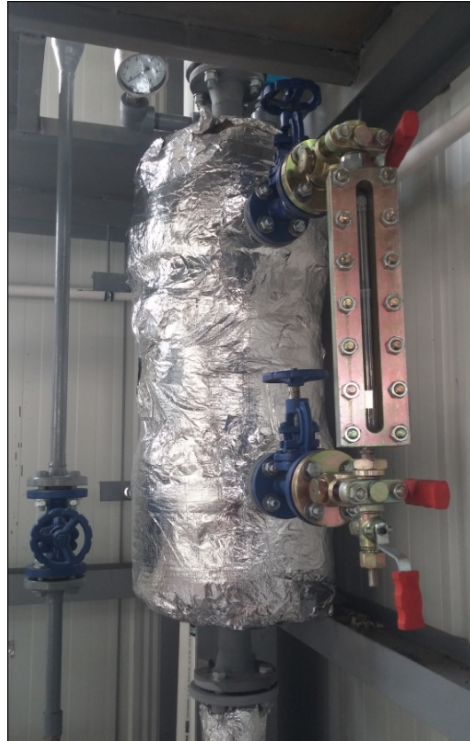
Figure 4.12. Installed expansion vessel on ORC test rig.
