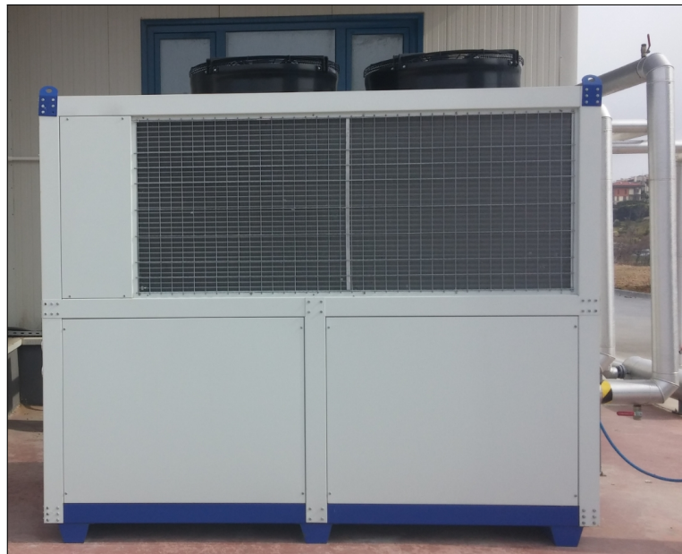
Figure 4.13. Installed chiller on ORC test rig.
