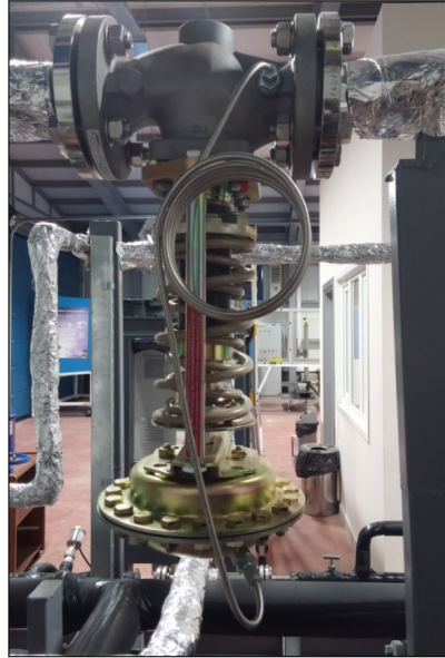
Figure 4.8. Installed throttle valve on ORC test rig.
