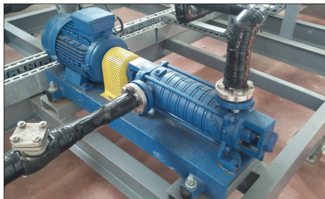
Figure 4.3. Installed side channel pump on ORC test rig.
