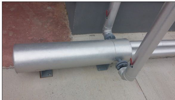
Figure 4.16. Installed fluid recovery exchanger on ORC test rig.
