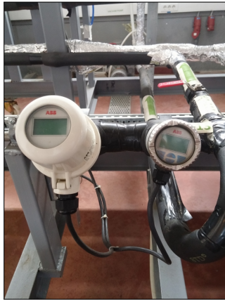
(a) Temperature (left) and pressure (right) transmitters
