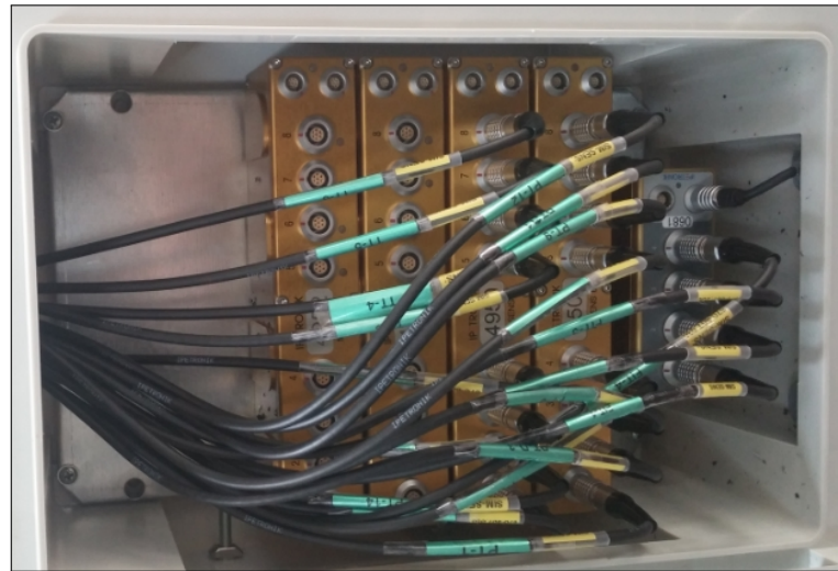
Figure 4.21. Installed M-SENS module on ORC test rig.
