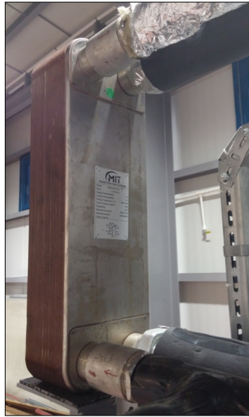
Figure 4.5. Installed brazed type heat exchanger on ORC test rig.
