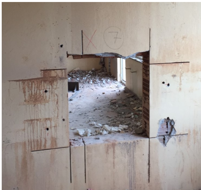
Figure 4.3. Gap in the partition wall due to extraction of the test specimen.
