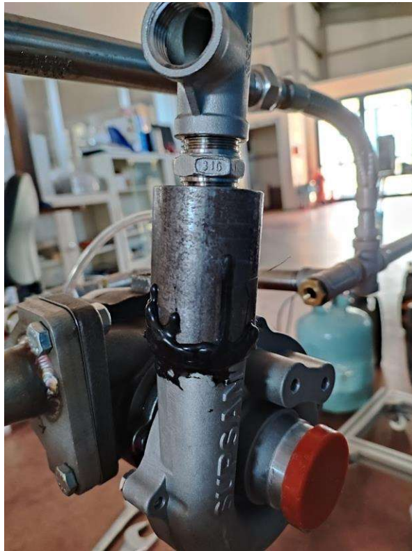
Figure 3.8. Compressor Outlet Connection.
