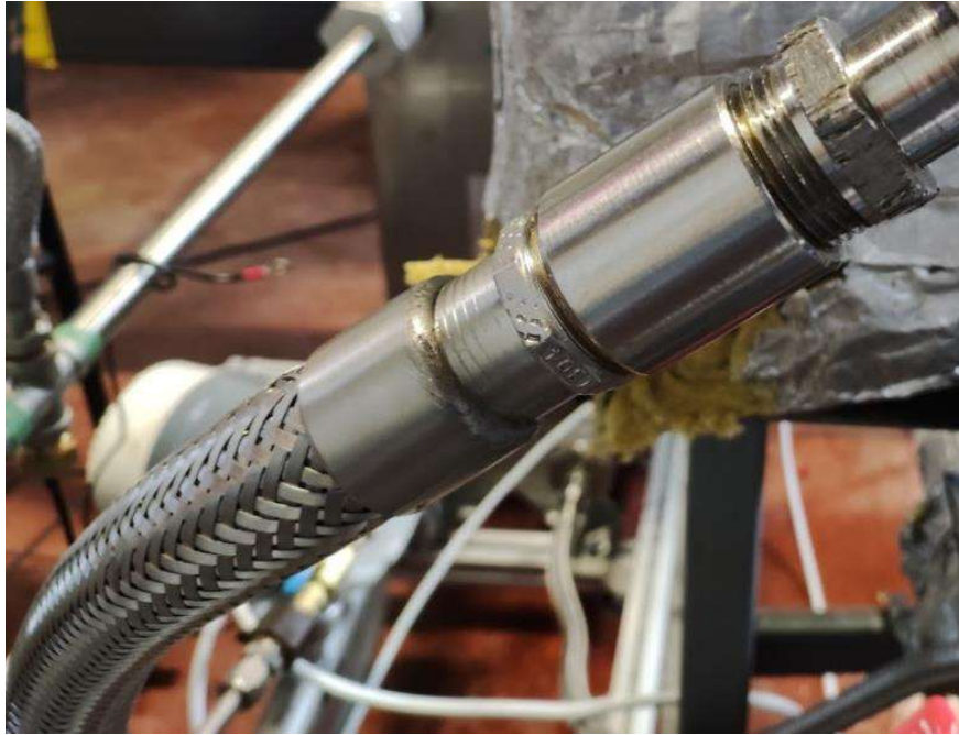
Figure 3.15. Flexible Pipe on Oil Line.
