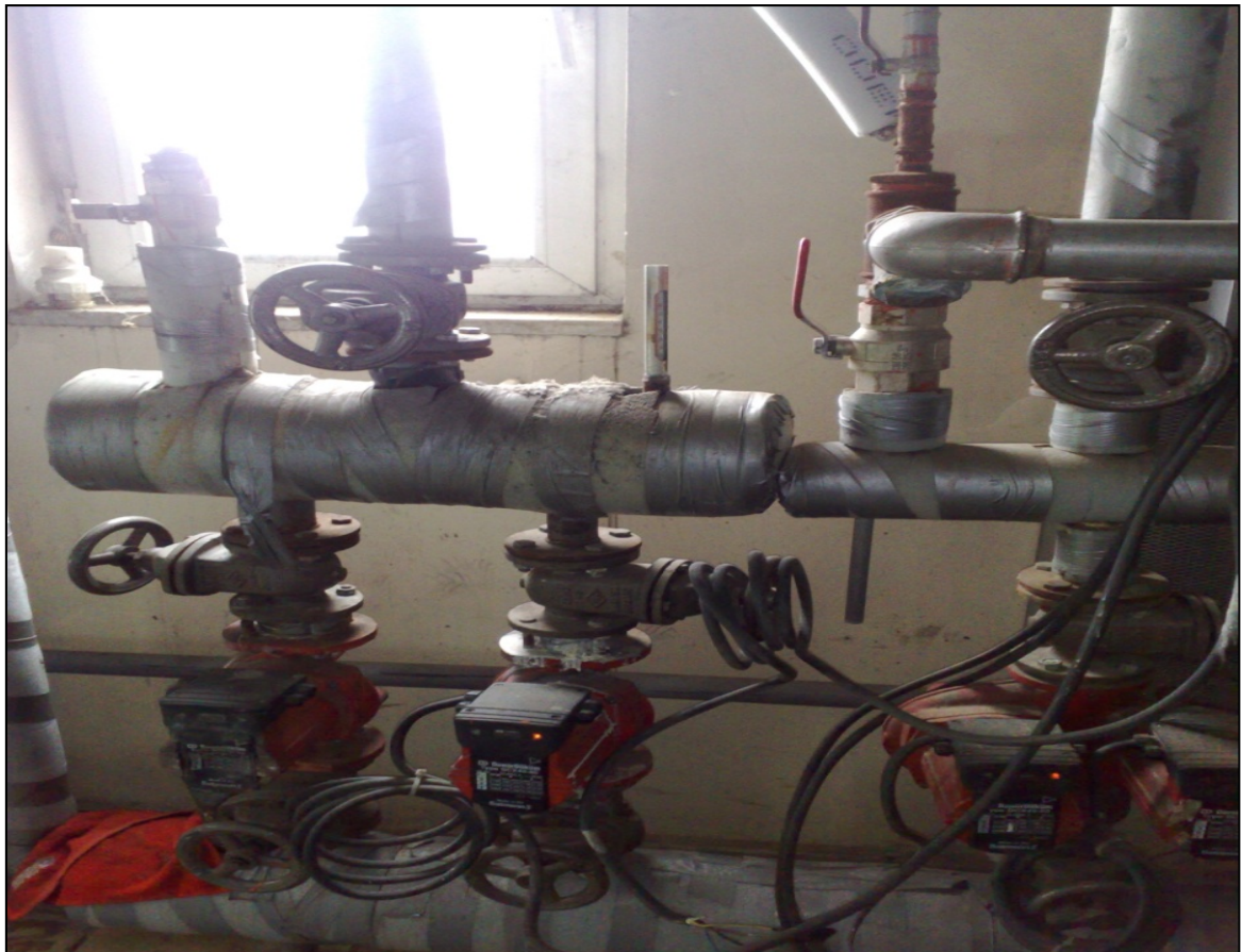
Figure 2.8. Heating System Valves.
