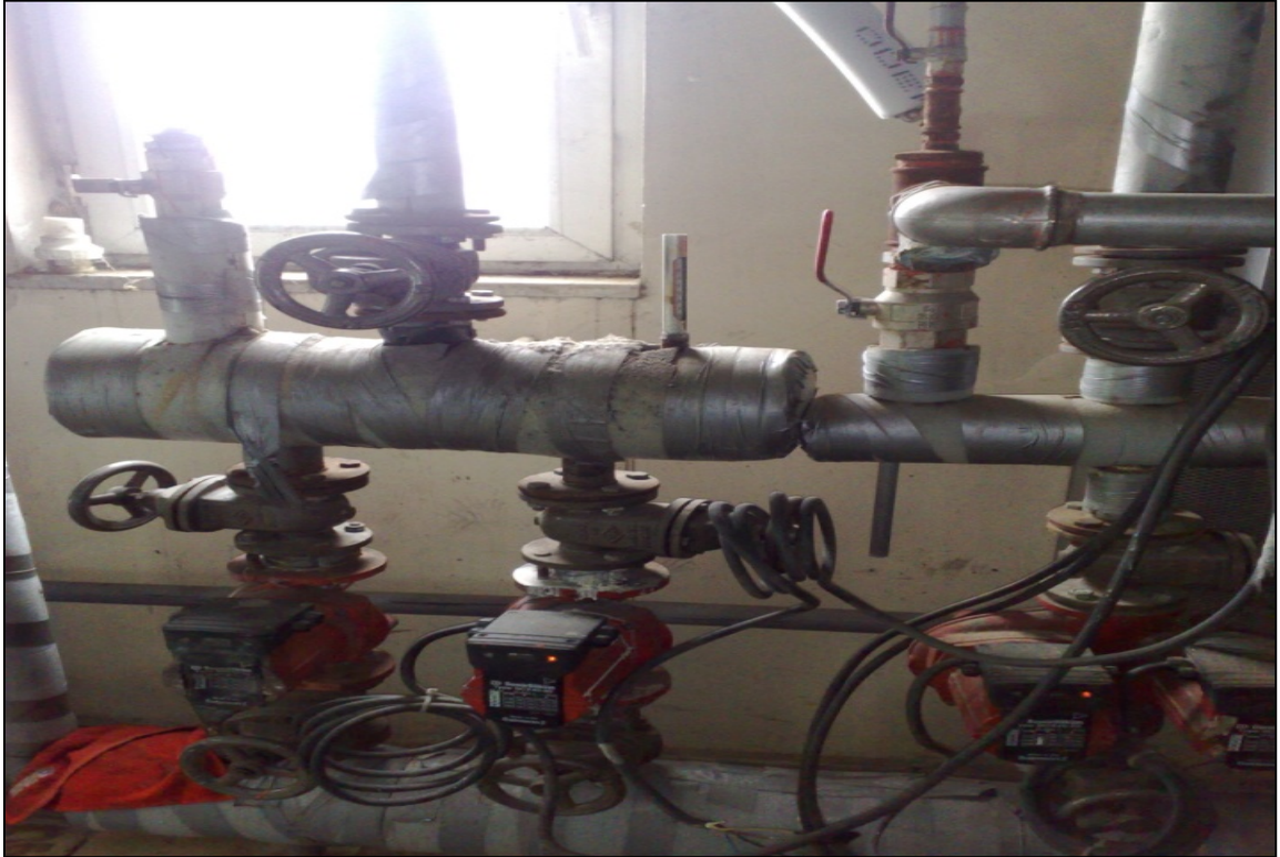
Figure 2.3. Heating System Pumps.
