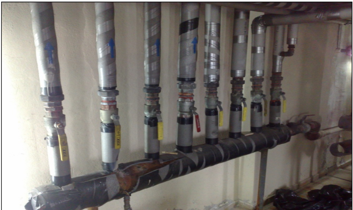
Figure 2.4. Heating System Piping.
