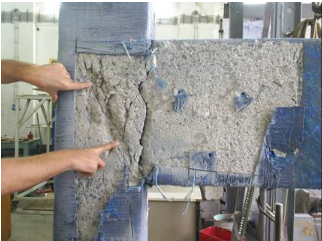
Figure 4.15. Damage at the joint region after removal of the CFRP sheets
