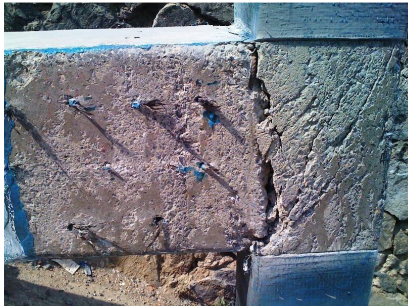
Figure 3.2. Main cracks after removing the CFRP sheets
