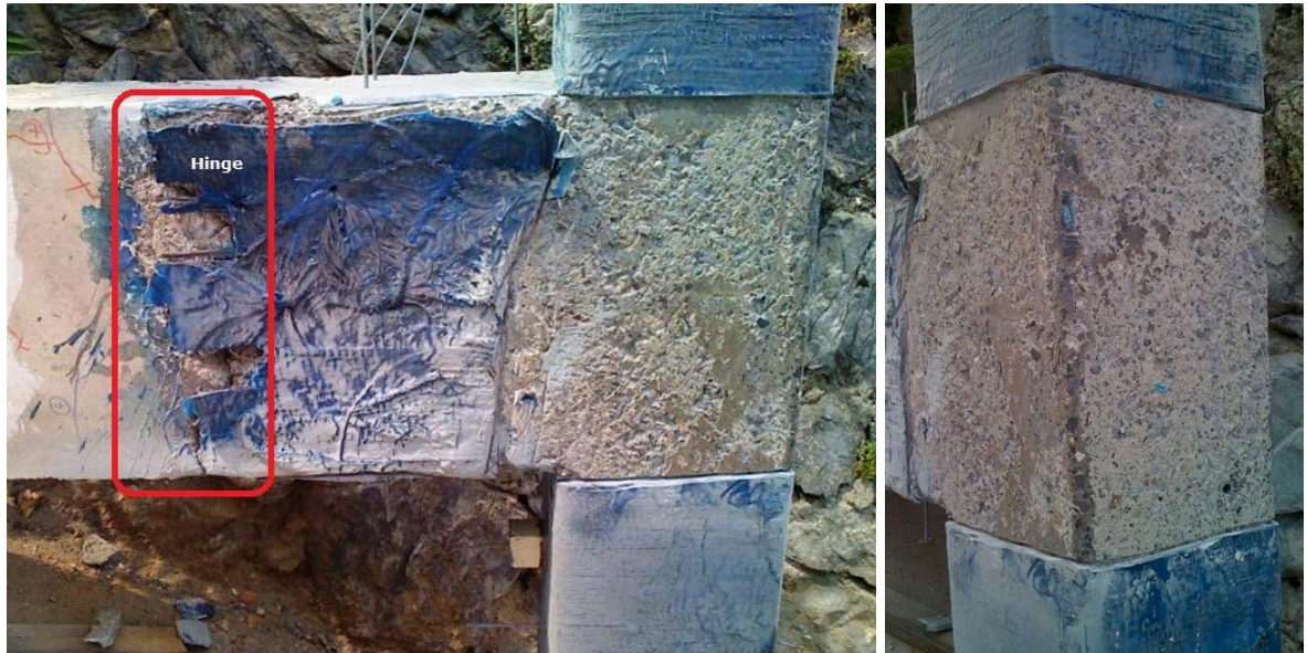
Figure 3.3. Hinge occurred in the beam and joint didn't crushed
