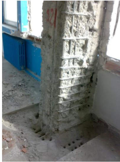
Figure 3.7. Existing Column with Cover Concrete Removed.
