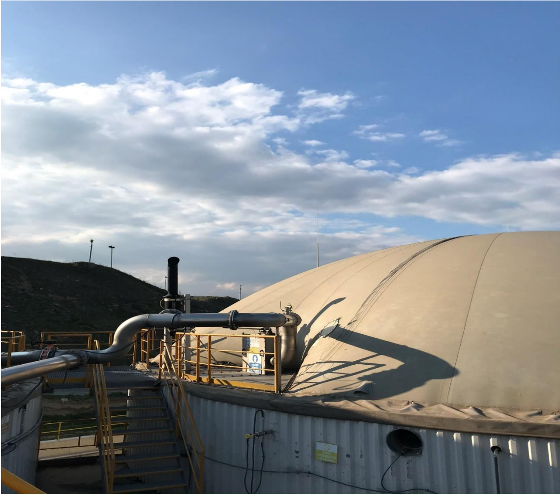
Figure B.5. Membrane biogas holder.
