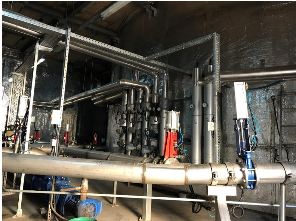
Figure B.10. The connections between the anaerobic reactors.
