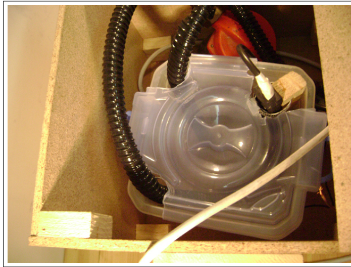
Figure 3.3 Inside of the hot water circulator
