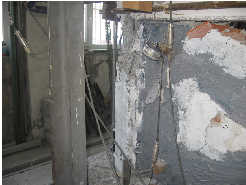
Figure 4.14. Beam-column joint failure for specimen O2
