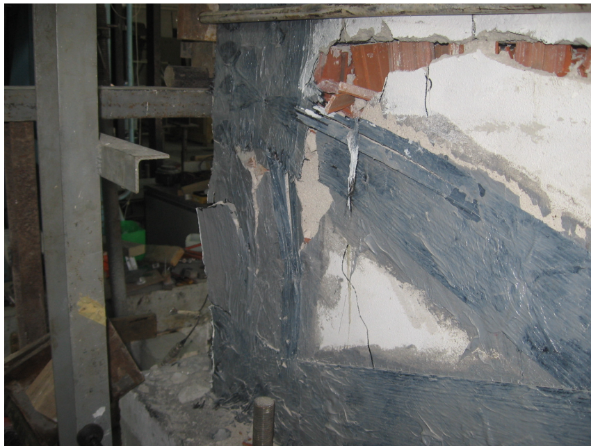
Figure 4.13. Rupturing of diagonal and vertical FRP for backside of specimen O2
