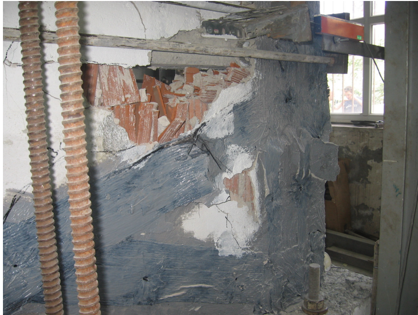
Figure 4.12. Rupturing of diagonal FRP for specimen O2
