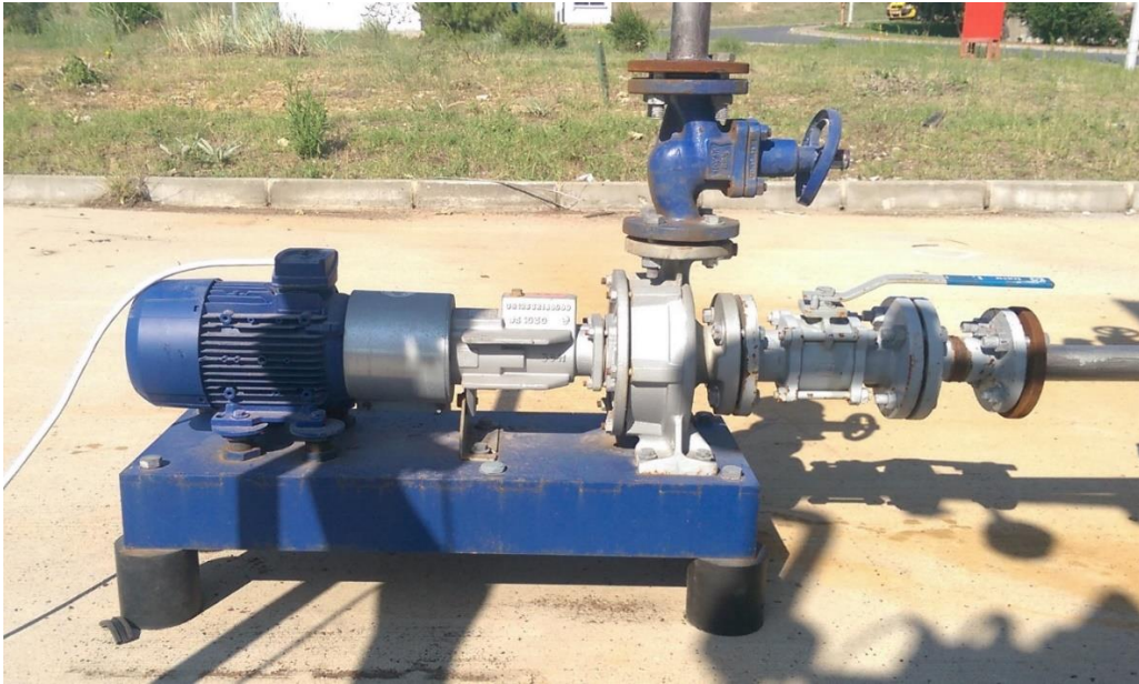
Figure 3.5. Oil circulation pump.
