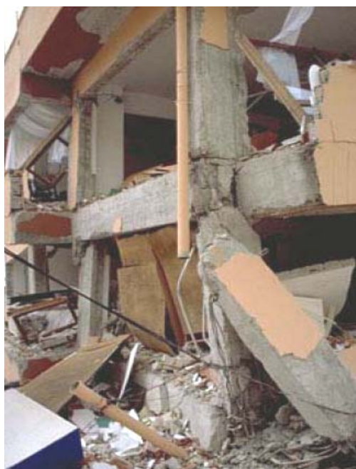
Figure 1.1. Joint failure from 1999 Kocaeli EQ (Sezen et al. , 2000)
