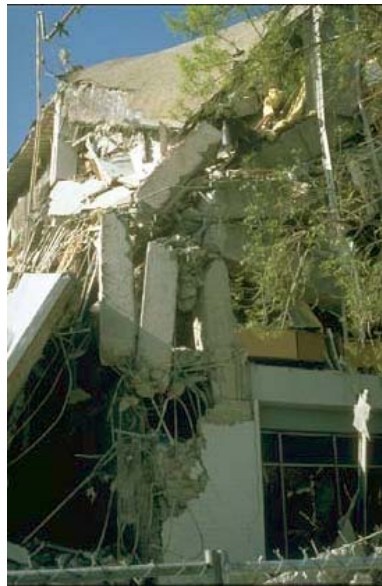
b) Typical Joint Failures
