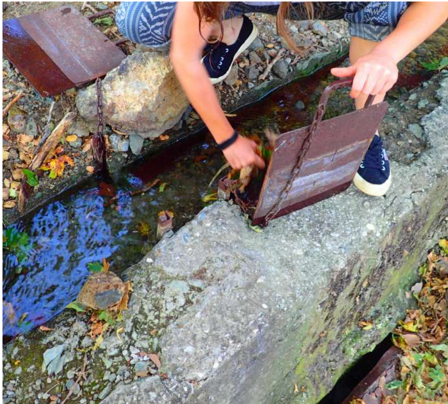
Figure 4.14. Sluice gate. The position of the panels directs the flow to the lower channel.
