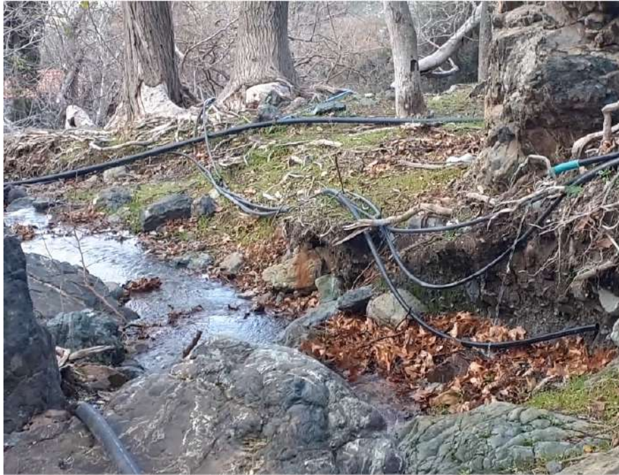
Figure 4.26. Redundant Pipes at Sotiras. Courtesy of Maria P.
