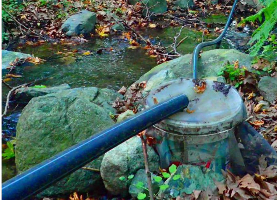
Figure 4.17. Improvised Filtration System.
