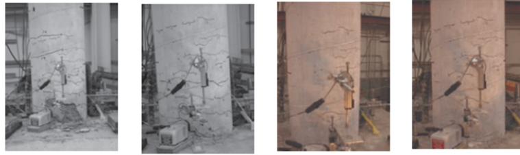
Figure 2.9. Damage observed on bent-1 after T13, T14, T15, T19; respectively (Johnson et al. , 2006).
