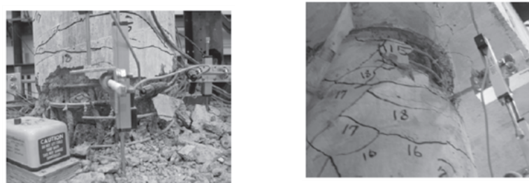
Figure 2.10. Damage observed on the lower and upper portion of bent-3 after T19 (Johnson et al. , 2006).
