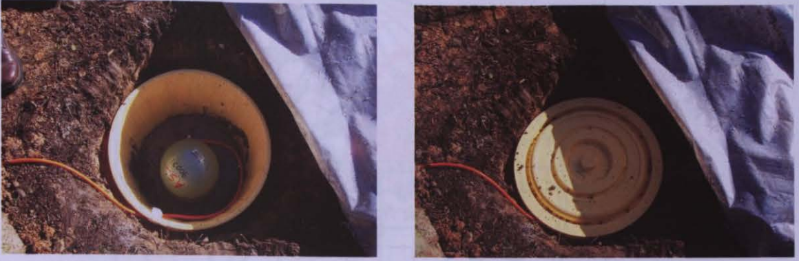
Figure 3.3 STS-2 seismometer is installed in a well and its upper part is covered by soil.
