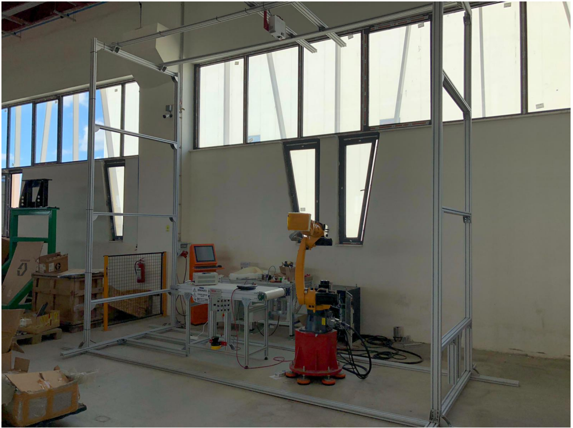
Figure 3.12. The robotic cell with all necessary components implemented in the HKTM A.Ş. production site.
