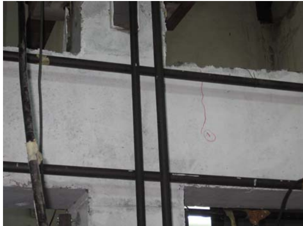
Figure 3.2. The first Flexural Cracks on Beam in Control Specimen
