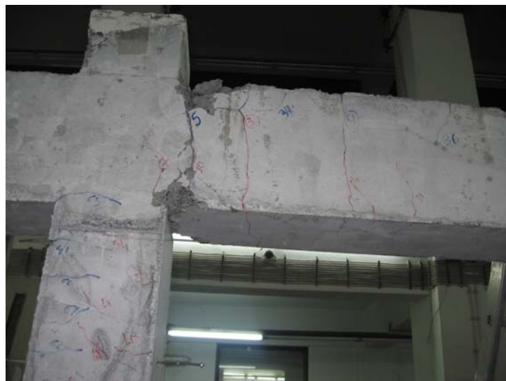
Figure 3.9. Crackings of Beam and Column at the end of the Test for Specimen LS
