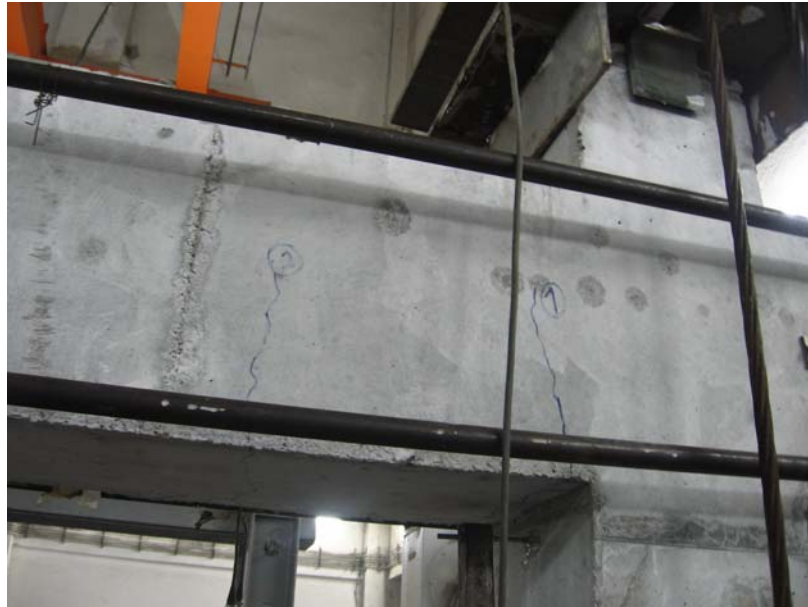
Figure 3.7. The First Flexural Cracks on the Beam in Specimen LS
