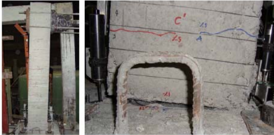
Figure 8.61. Damage at the Base of Specimen LS-55φ-N1 (Yilmaz, 2009).
