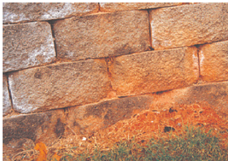
Figure 4.35. An example of reinforced soil flowing from block due to water infiltrating at the top of a wall (Narejo and Ramsey, 2001).
