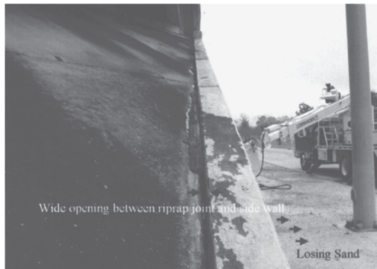
Figure 4.37. Wide opening between riprap joint and sidewall permits water to enter riprap. Water carries sand through breached or rupture filter fabric (Chen et al. , 2007).
