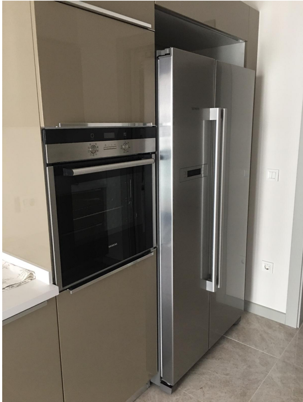
Figure 4.2. Building A kitchen oven.
