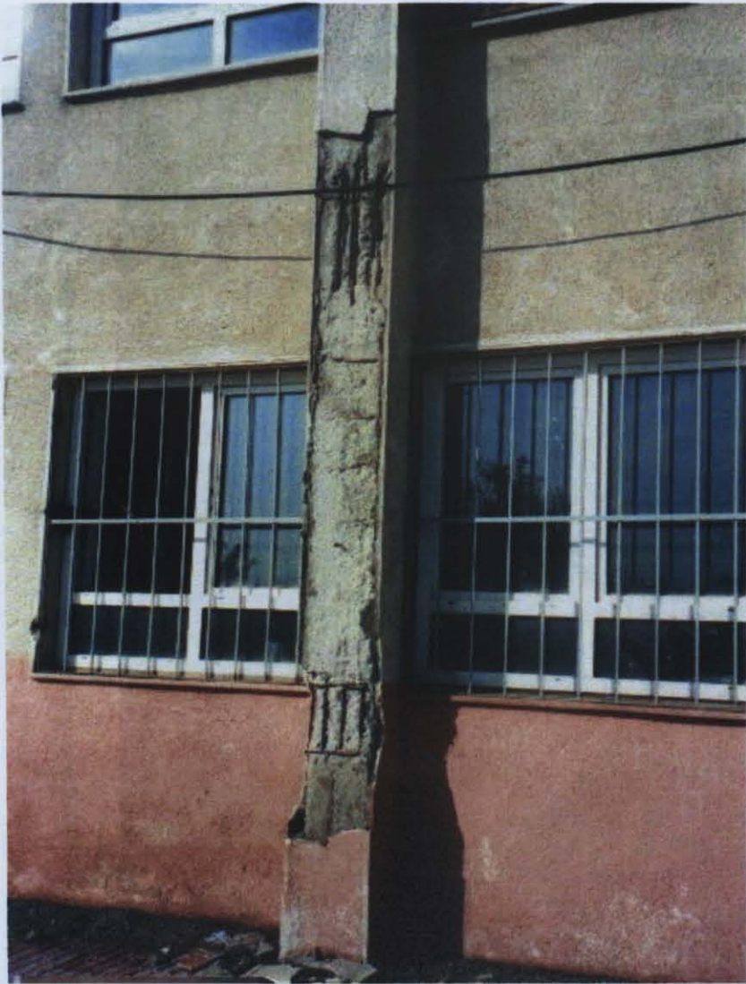
Photo D.23 – Lack of confinement at column at Ümraniye Genç Osman İ.Ö.O.
