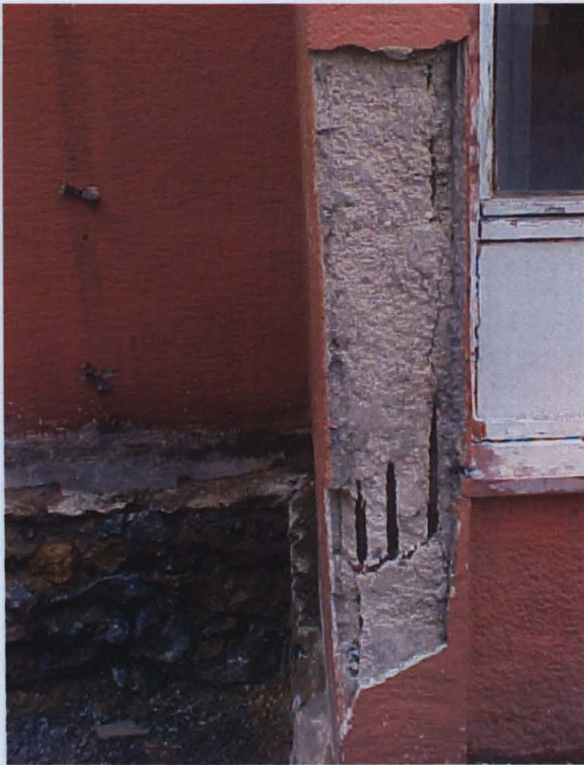
Photo D.29 – Corrosion of reinforcing bars with poor quality of reinforced concrete at Zeytinburnu Yedikule İ.Ö.O.
