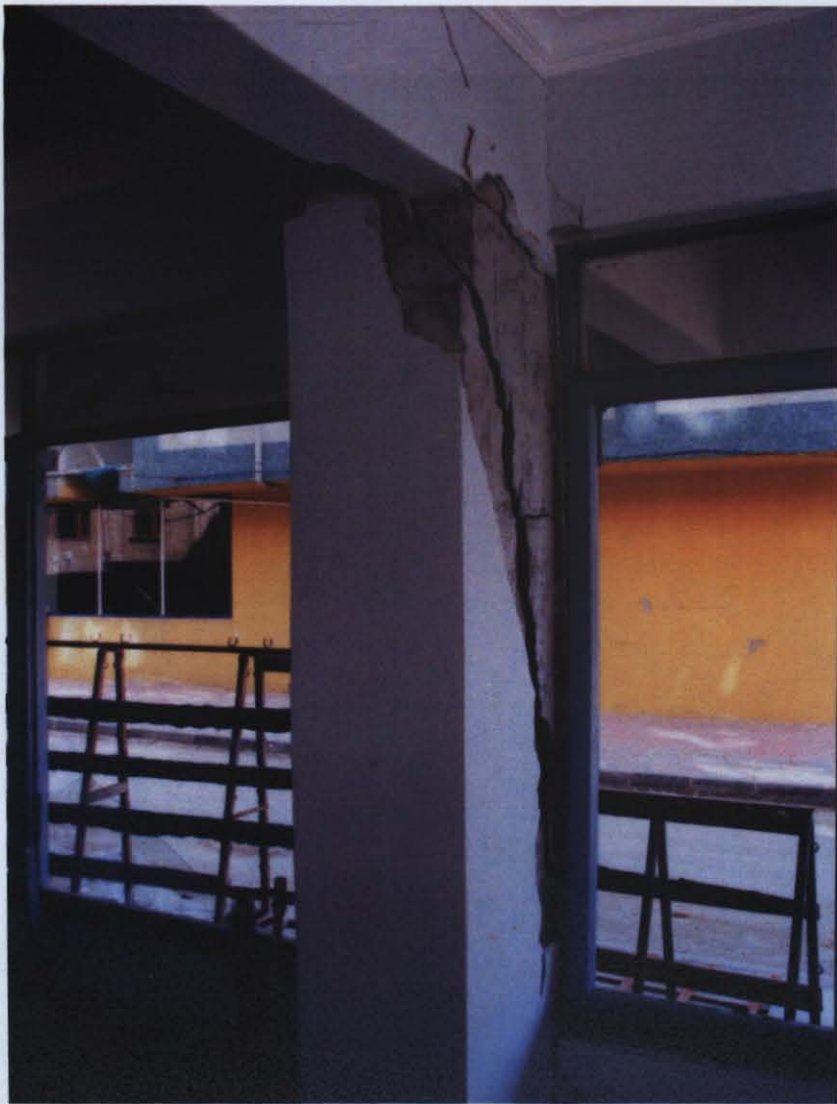
Photo D.31 – Heavy damaged column with shear crack
