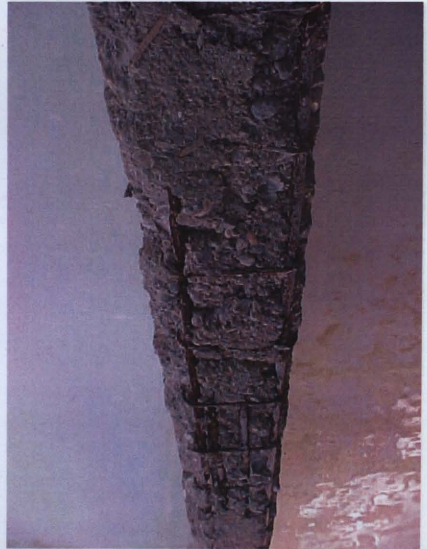
Photo D.10 – Lack of confinement and concrete strength problem at Fatih Kırımlı Aslanbey İ.Ö.O.
