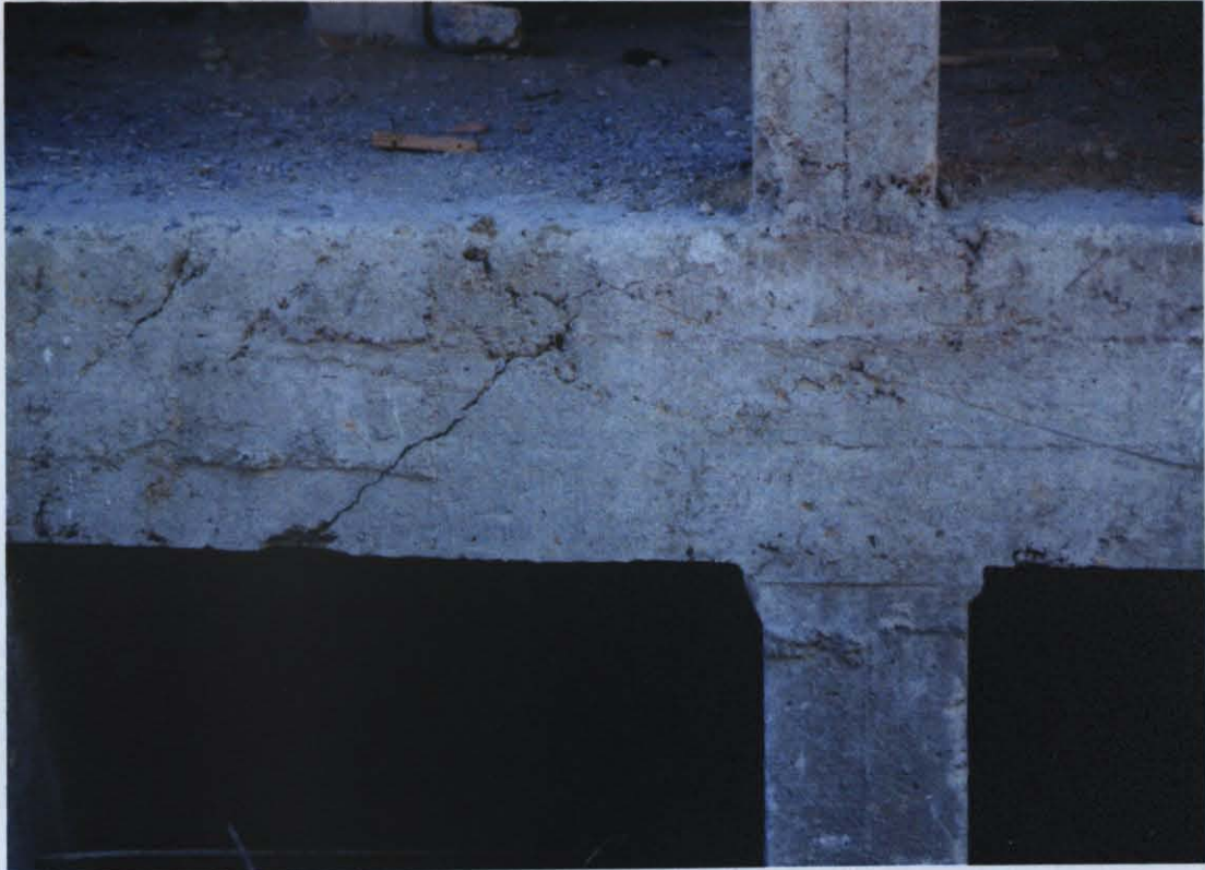
Photo D.6 – Shear crack at beam at Sarıyer Şükrü Nail İ.Ö.O.
