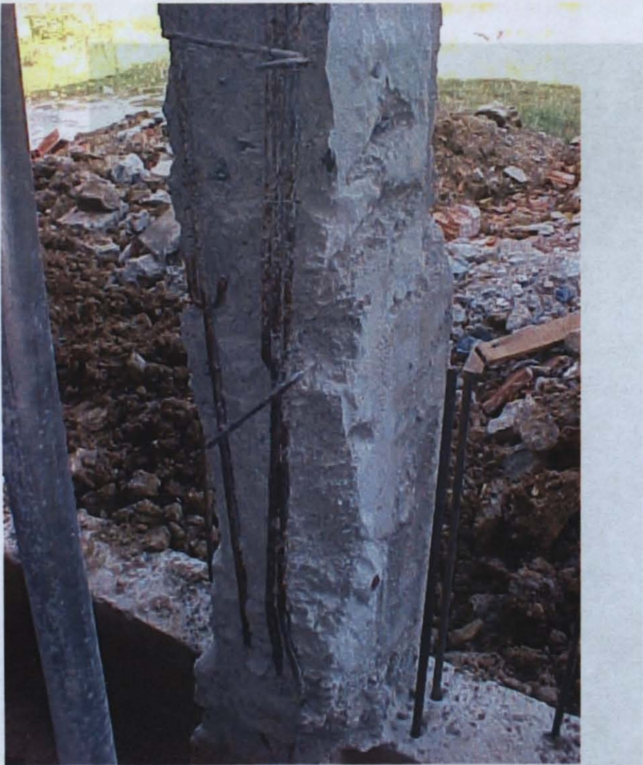
Photo D.1 – Unconfined concrete problem at Beykoz Dereseği İ.Ö.O.
