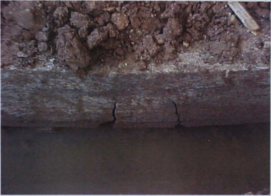
Photo D.19 – Shear crack in basement at Küçükçekmece Yunus Emre İ.Ö.O.
