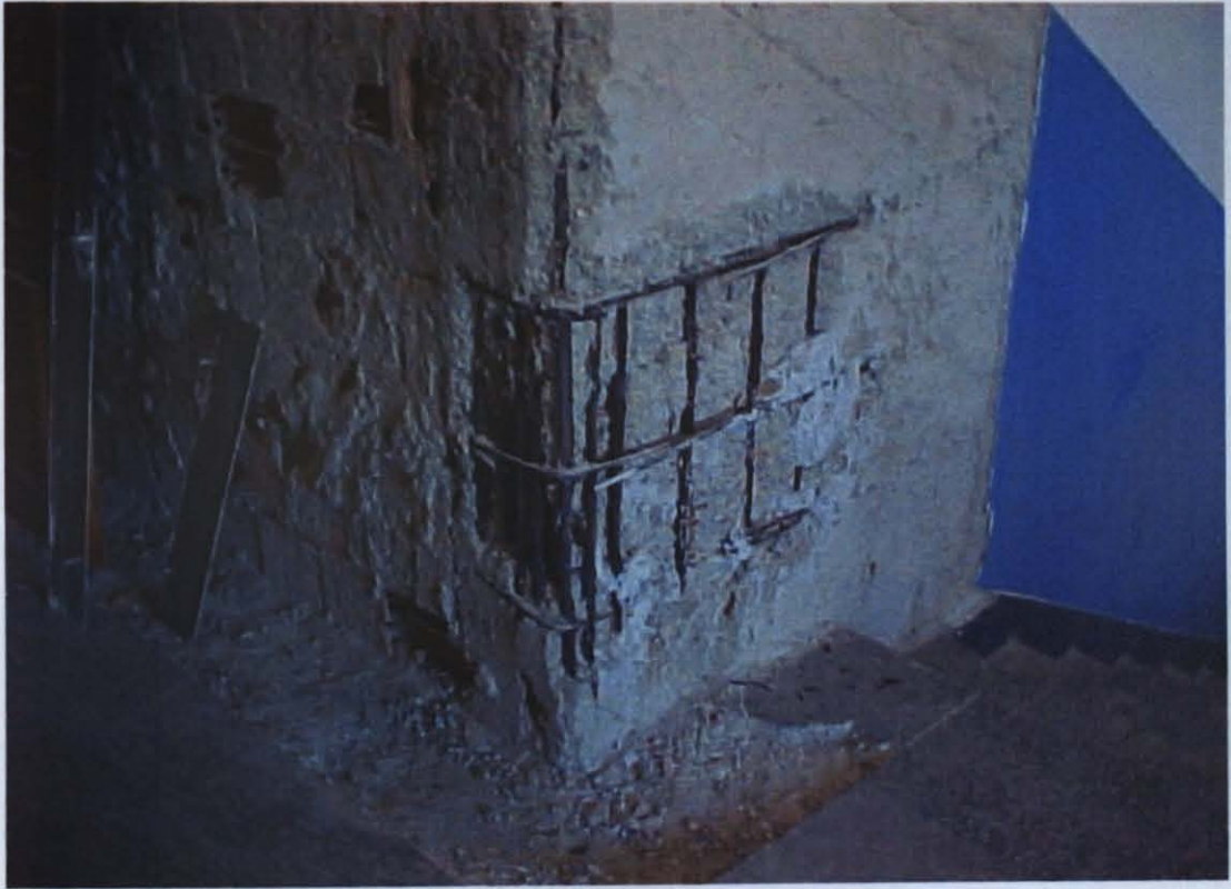
Photo D.16 – Concrete spalling at column end at Kartal Anadolu Lisesi
