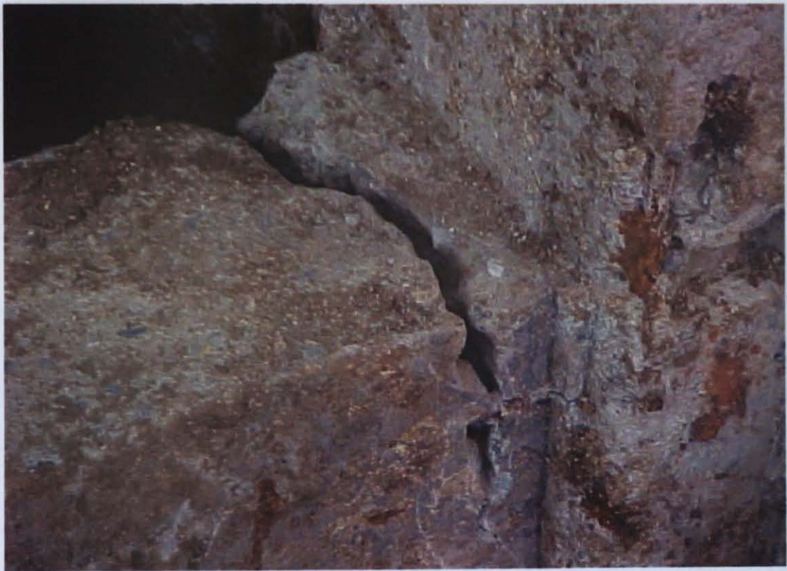
Photo D.18 – Close up of bending crack on tie beam at Küçükçekmece Yunus Emre İ.Ö.O.
