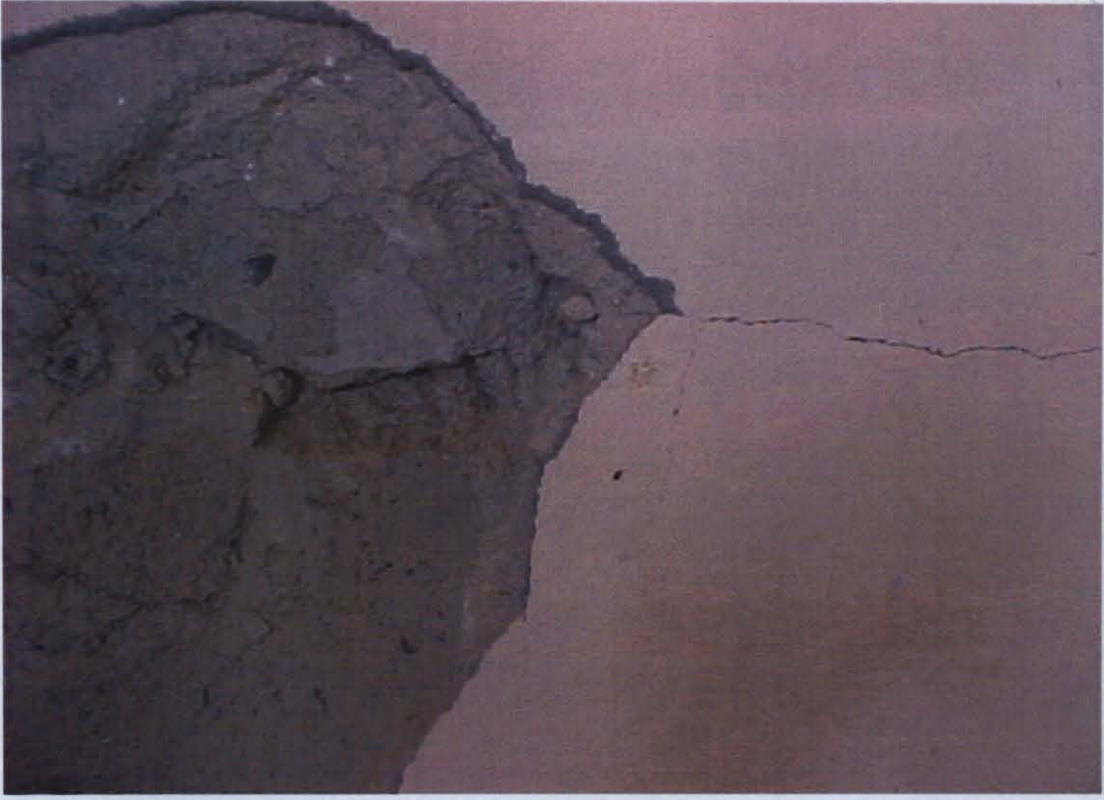
Photo D.5 – Heavy damaged shear wall crack at Büyükçekmece Gürpınar İ.Ö.O.
