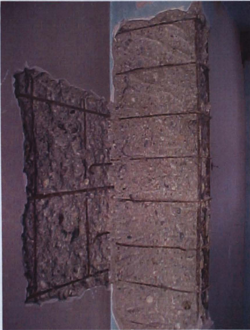
Photo D.9 – Corrosion problem and lack of confinement at Fatih Kırımlı Aslanbey İ.Ö.O.
