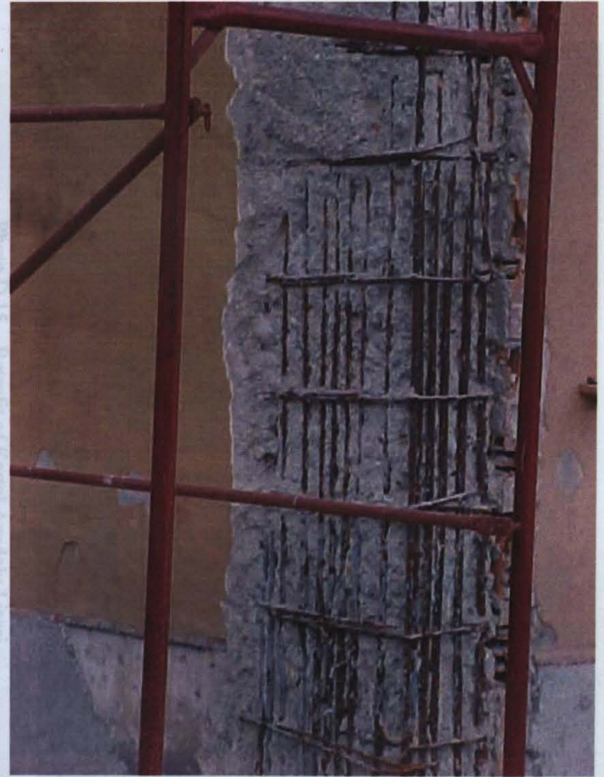
Photo D.14 – Bar density and concrete quality problem at Kartal Anadolu Lisesi
