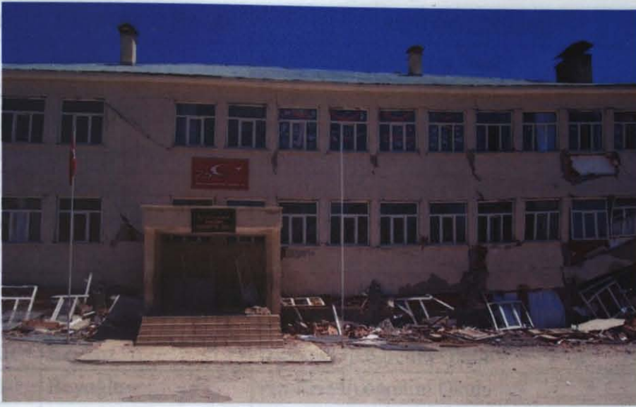
Photo 2.11 – Kaleönü İlköğretim Okulu collapsed after Bingöl earthquake
