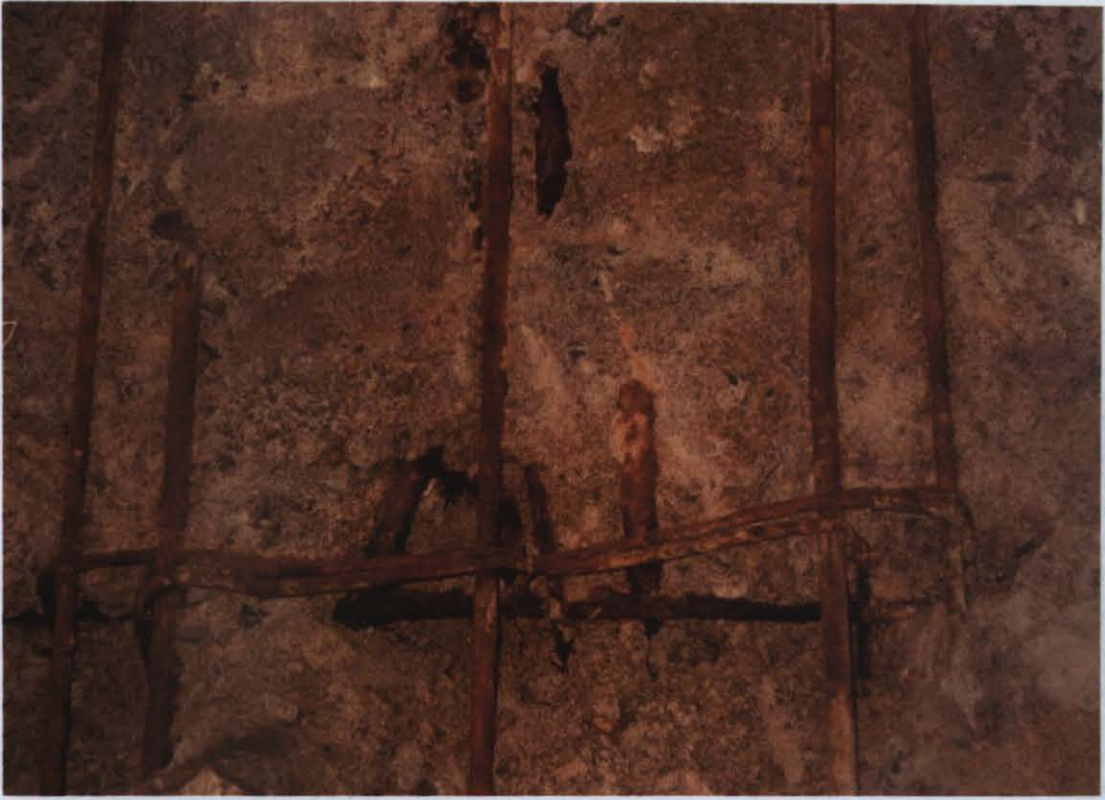
Photo D.33 – Corrosion problem and lack of confinement
