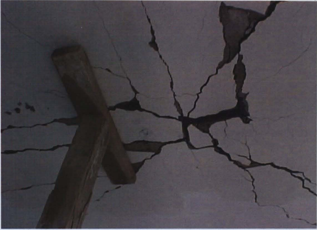
Photo D.3 – Cracks at slab and deflection problem at Büyükçekmece Gürpınar İ.Ö.O.
