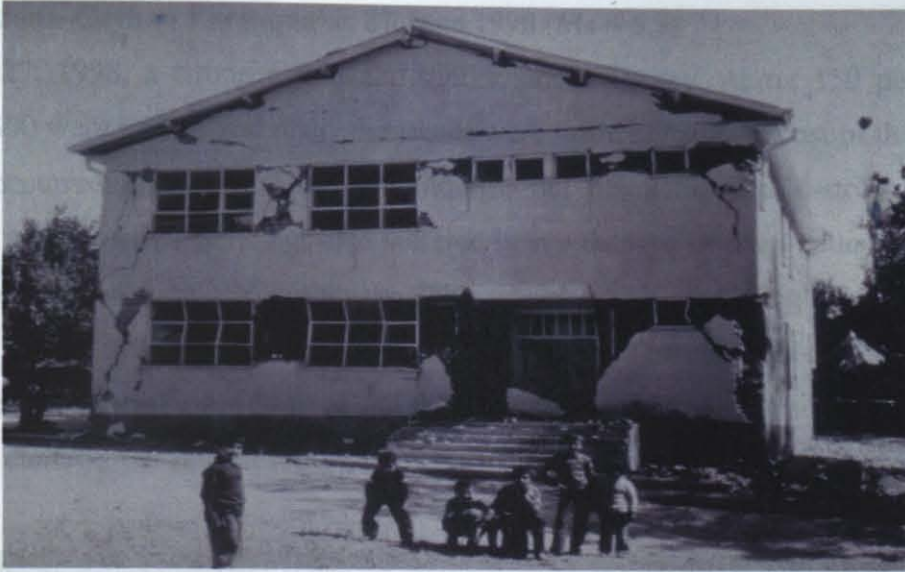
Photo 2.6 – Shear failure and cracked walls at Lice Secondary School
