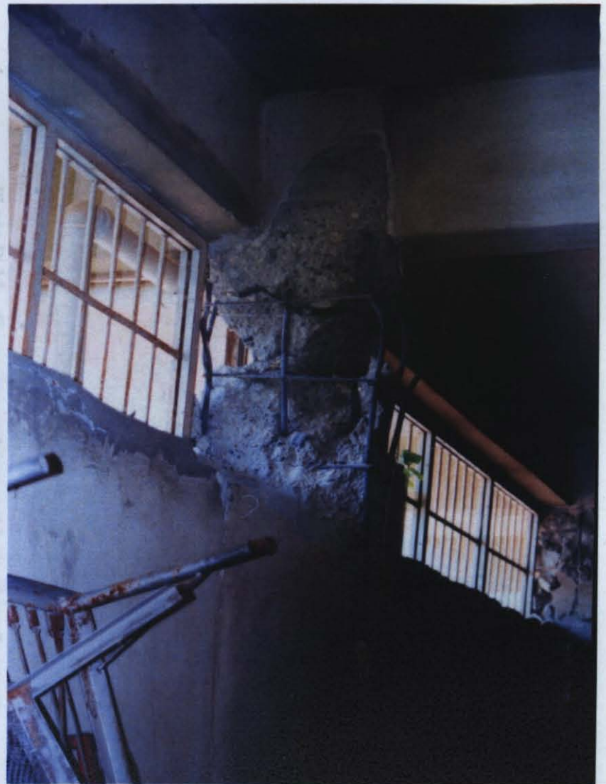
Photo D.32 – Short column effect with lack of confinement
