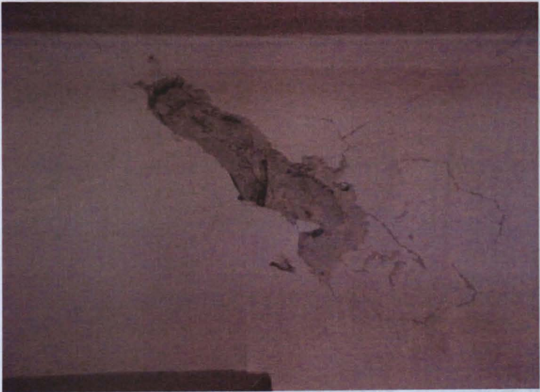
Photo D.20 – Heavy damaged shear wall at Küçükçekmece Yunus Emre İ.Ö.O.
