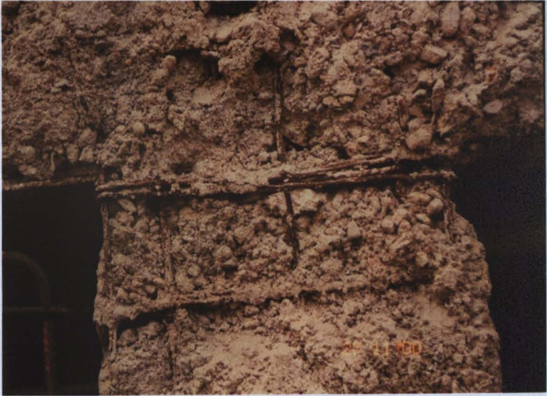
Photo D.34 – Corrosion problem, poor quality concrete and lack of confinement
