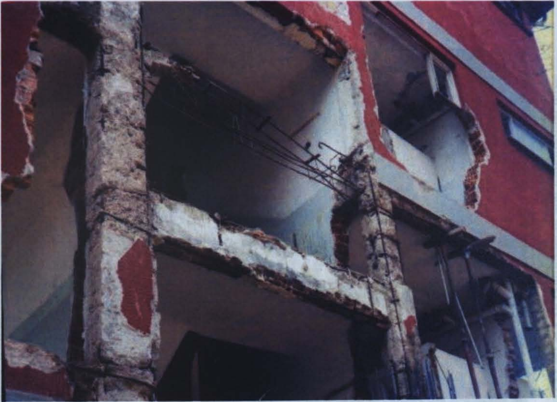
Photo D.26 – Insufficient structural design with poor detailing at Üsküdar Halil Rüşti İ.Ö.O.
