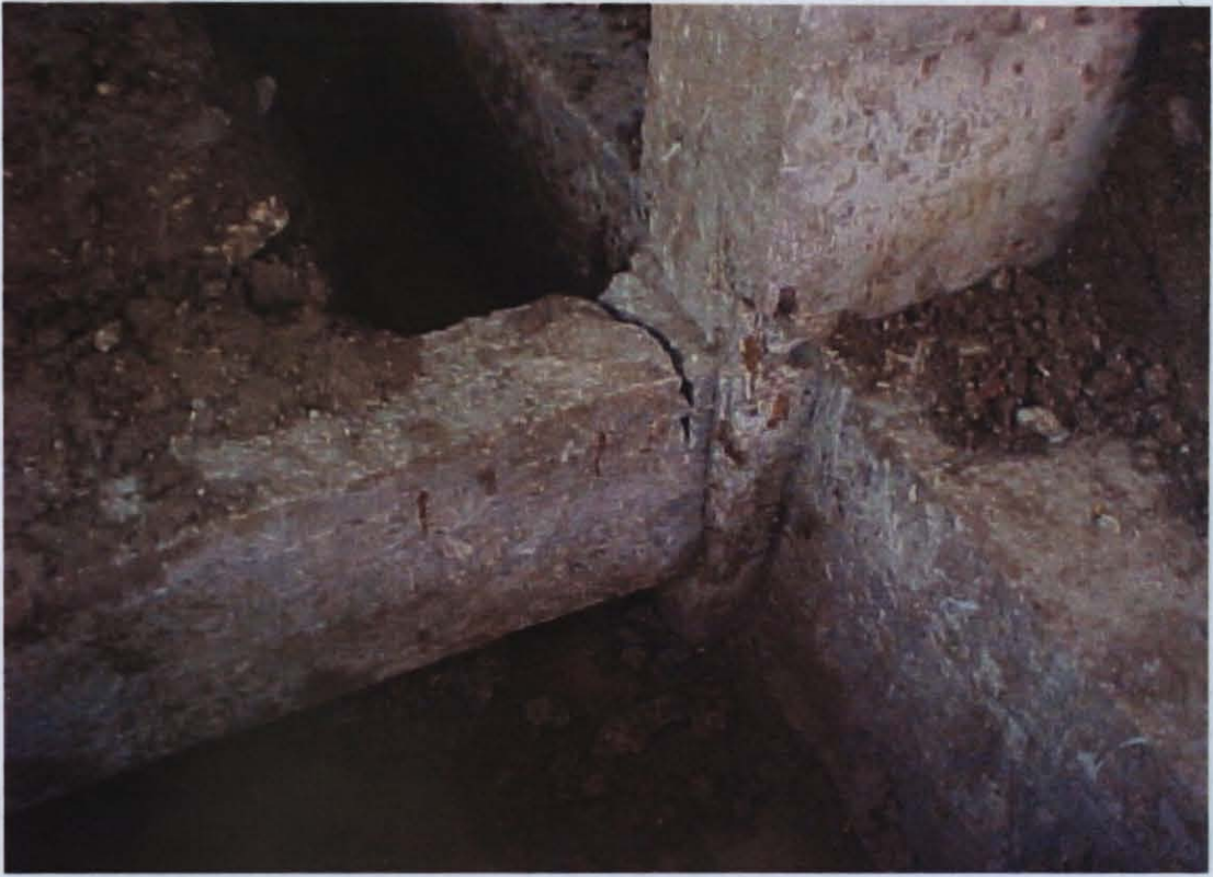
Photo D.17 – Bending crack on tie beam at Küçükçekmece Yunus Emre İ.Ö.O.
