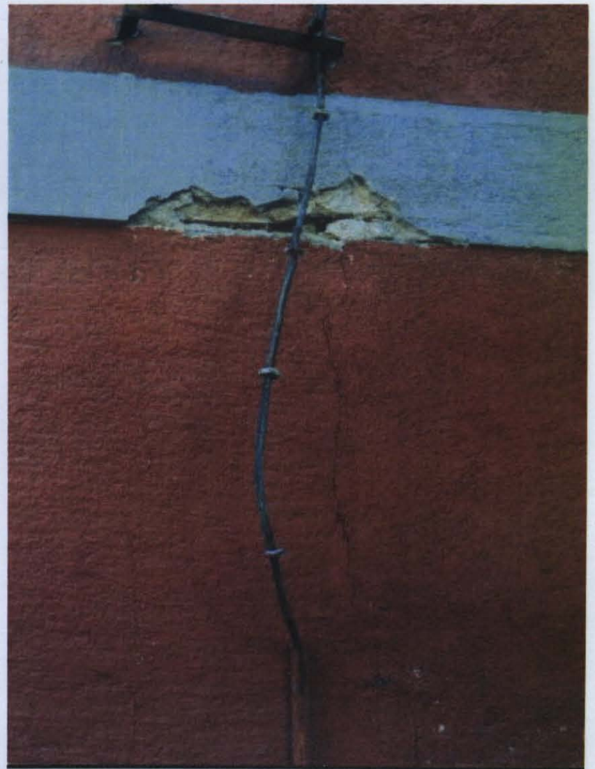
Photo D.28 – Crack on infill walls and corrosion problem at Üsküdar Halil Rüştü İ.Ö.O.
