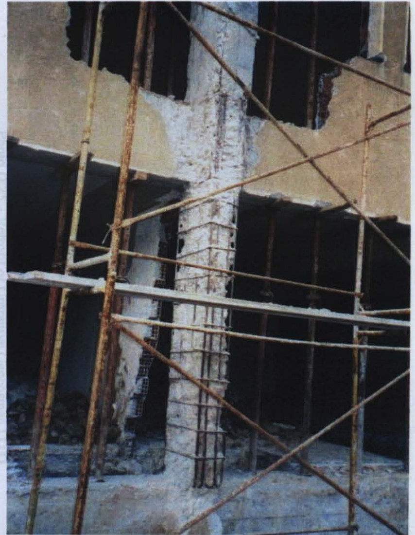
Photo D.24 – Lack of confinement and retrofit of Ümraniye Genç Osman İ.Ö.O.
