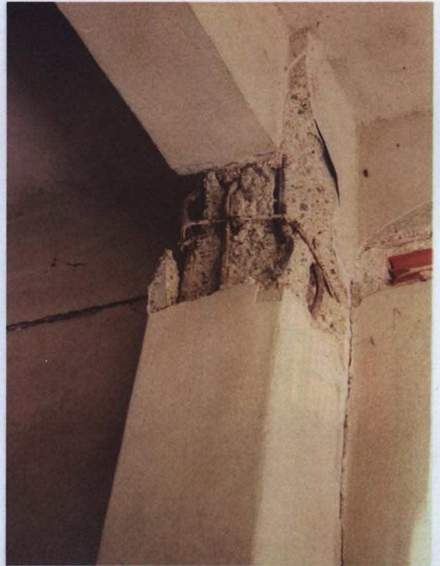
Photo D.30 – Failure of column/beam connection with buckling of longitudinal bar due to poor confinement Zeytinburnu Yedikule İ.Ö.O.
